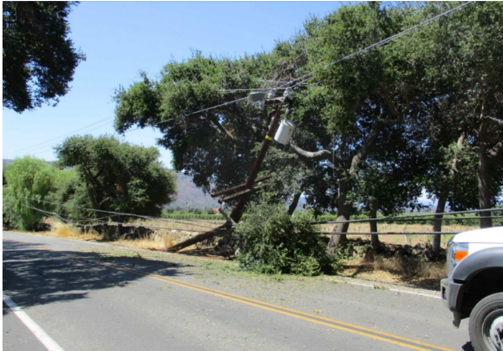
Figure SCE 9.10-5 Covered Conductor Contact with Vegetation After Car-Hit-Pole Ojai, California – July 24, 2020
