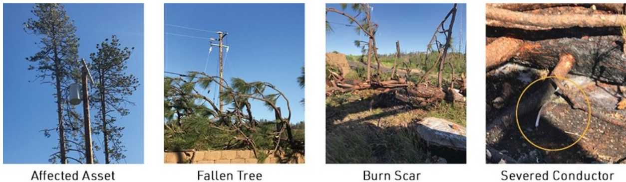
Figure CC-2 PG&E Covered Conductor Effectiveness – Example 1
