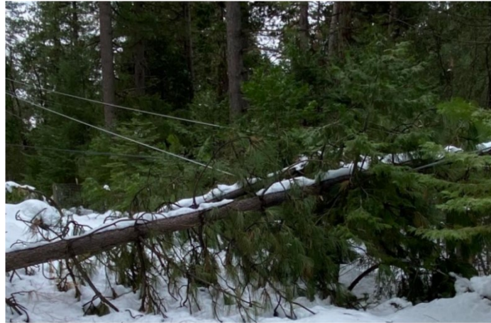
Figure CC-4 PG&E Covered Conductor Effectiveness – Example 3
