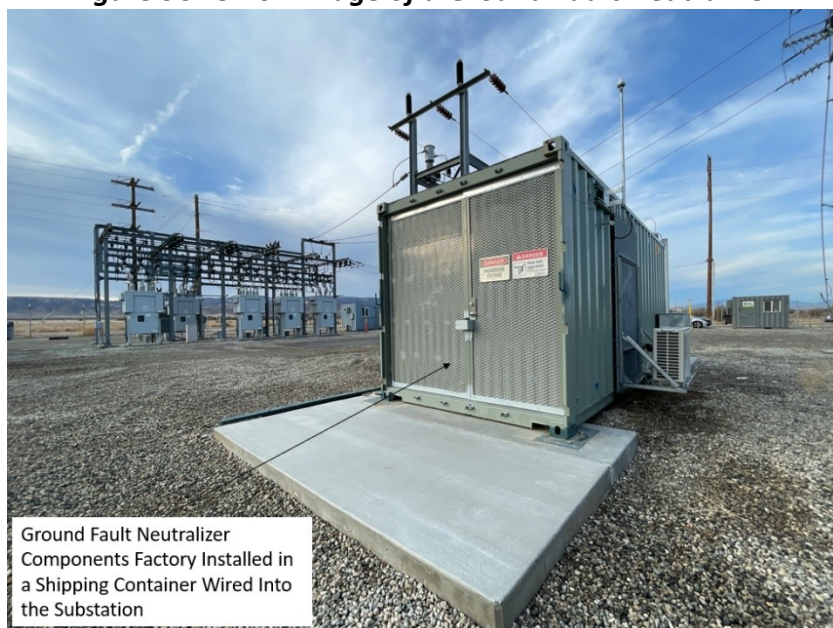
Figure SCE 8-10 - Image of a Ground Fault Neutralizer
