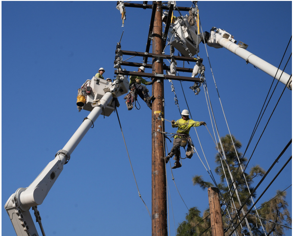
As High Fire Risk Areas expand, SCE is evolving our Public Safety Power Shutoff program to help keep communities safe.
