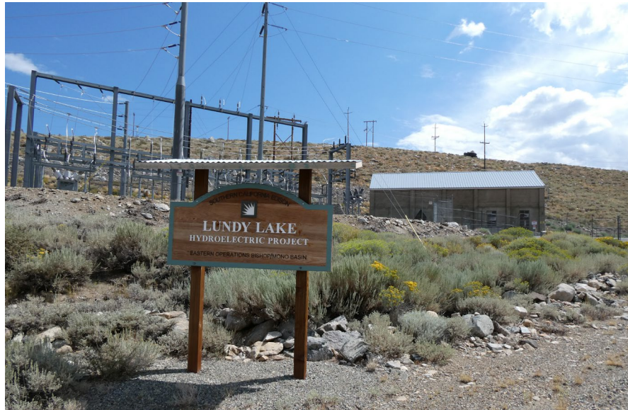
Powerhouse and switchyard, Lundy Lake Hydroelectric Project, camera facing southeast, August 2025.
