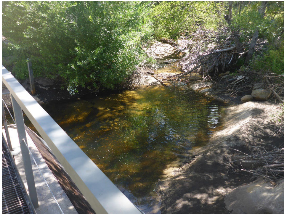
Figure A-46. Minor sand and debris accumulation on the upstream face of Corral Creek Diversion Dam.
