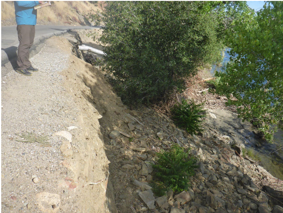
Figure A-66. Potential erosion of road prism fill near KR3 Powerhouse access road and gate.
