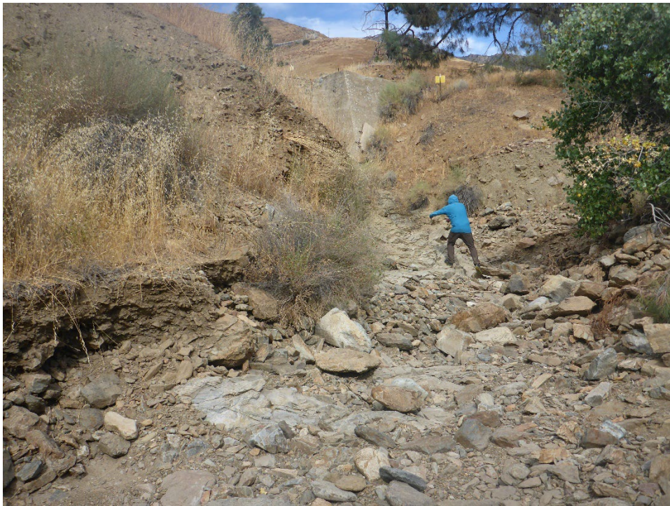
Figure A-62. KR3 Powerhouse Forebay Spillway channel where it empties into the Kern River floodplain (looking upstream).
