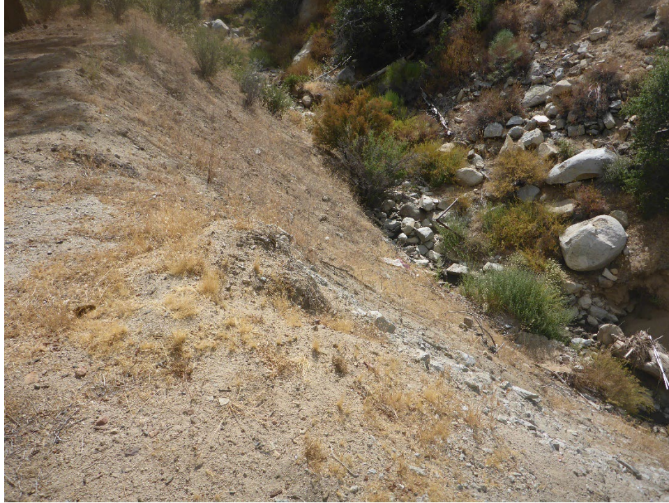
Figure A-7. Historical tunnel spoil material placed in drainage swale at Tunnel 4/5 Spoil Site (view looking into channel from downstream margin of spoil pile).
