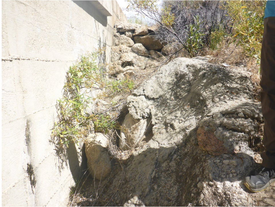
Figure A-45. Gunite erosion control/bank stabilization along upstream edge of Corral Creek crossing flume.
