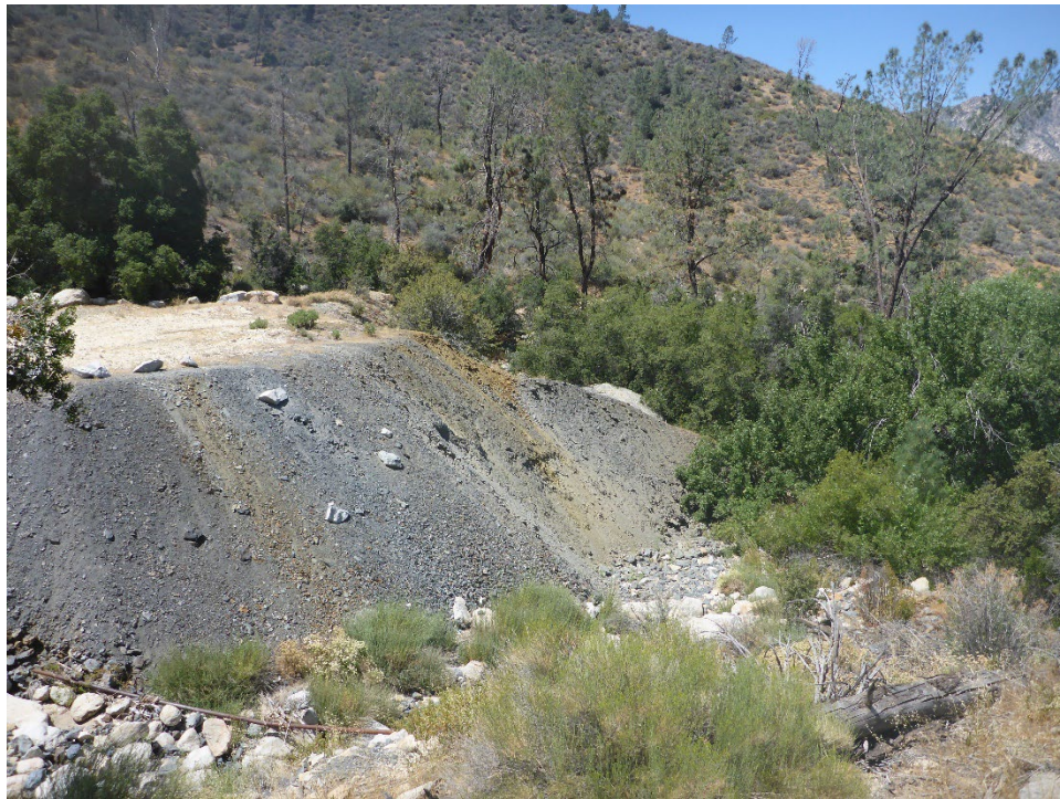
Figure A-48. Moderate erosion of left bank (south side) of Corral South Tunnel 18 Spoil Site; sediment delivered directly to the watercourse.
