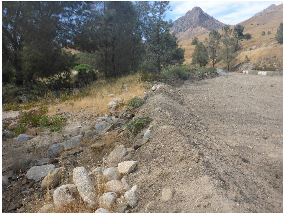
Figure A-64. Small berm constructed of sediment and debris from the March 2023 flood event deposited at the KR3 Powerhouse maintenance yard.
