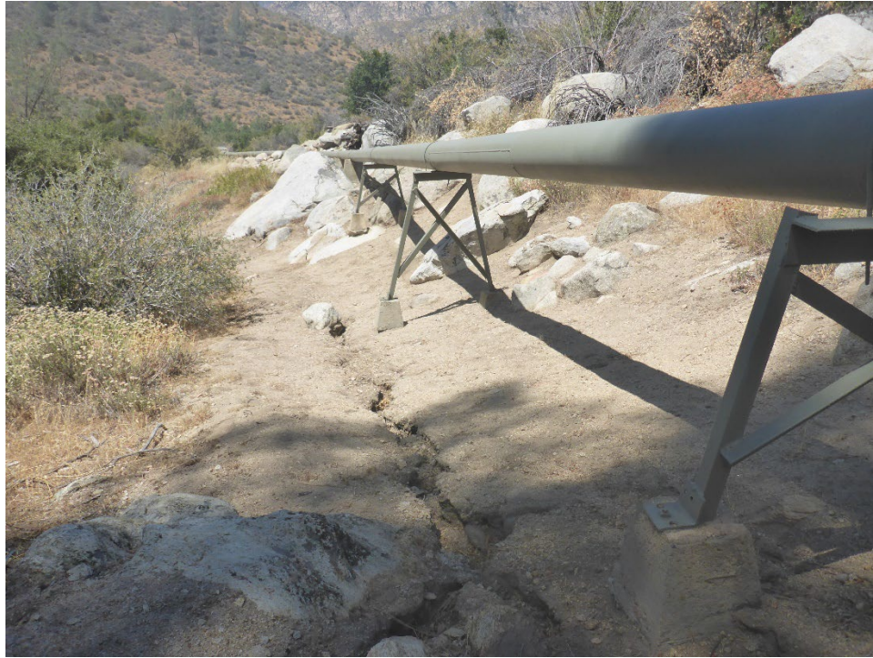
Figure A-47. Small gully erosion along Corral Creek Diversion Tunnel, approximately 300 feet upslope of point where diversion empties into exposed tunnel structure.
