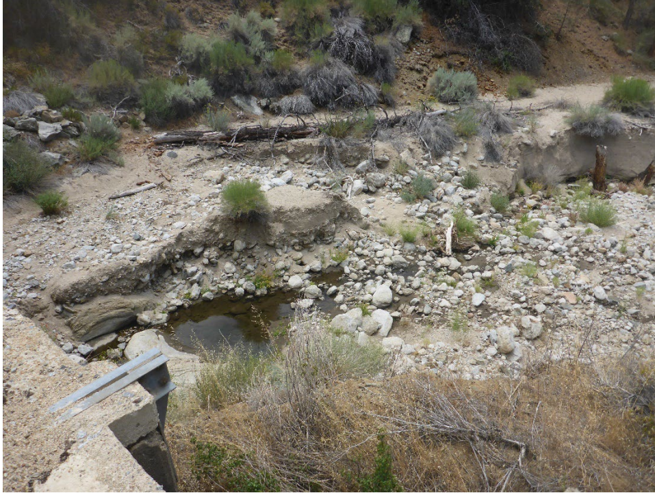
Figure A-25. Close-up view of failed road Crossing at Tunnel 9B/10 Spoil Site (view looking across channel at left bank [south side]).
