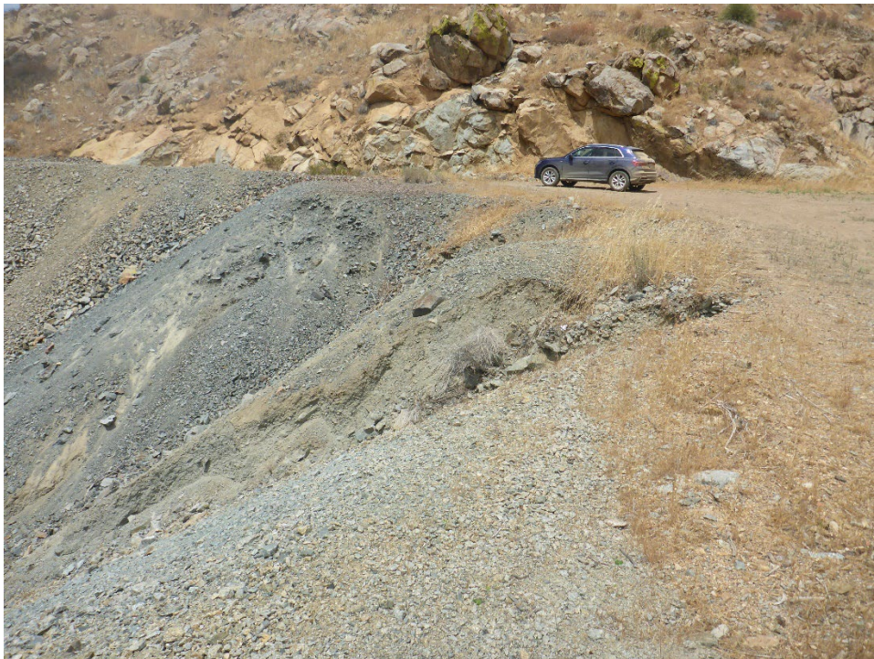
Figure A-36. Moderate erosion of coarse spoil material placed in steep drainage swale at Tunnel 14 Spoil Site; sediment delivered directly to watercourse.
