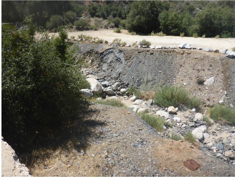
Figure A-49. Additional view of moderate erosion along left bank (south side) of Corral South Tunnel 18 Spoil Site (view immediately adjacent to left of Figure A-48 image).
