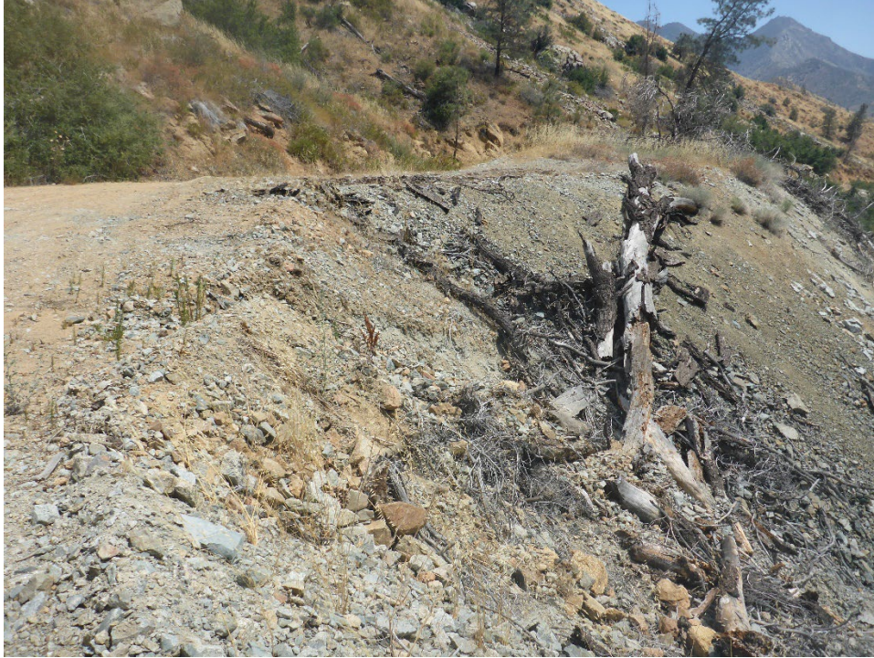
Figure A-33. Close-up view of access road built on top of Tunnel 12/13 spoil material (Figure A-32 image immediately adjacent to right side of Figure A-33 image).
