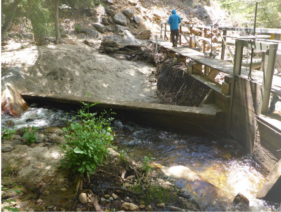
Figure A-19. Upstream side of Salmon Creek Diversion Dam with sand and debris accumulation above Diversion intake structure (view from right bank toward left bank, north to south).
