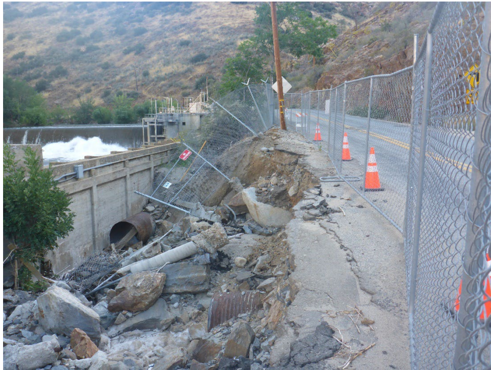
Figure A-1. Erosion of (non-Project) Mountain Highway 99 at Fairview Dam Sandbox Facility initiated by failed culvert crossing (view looking upstream).
