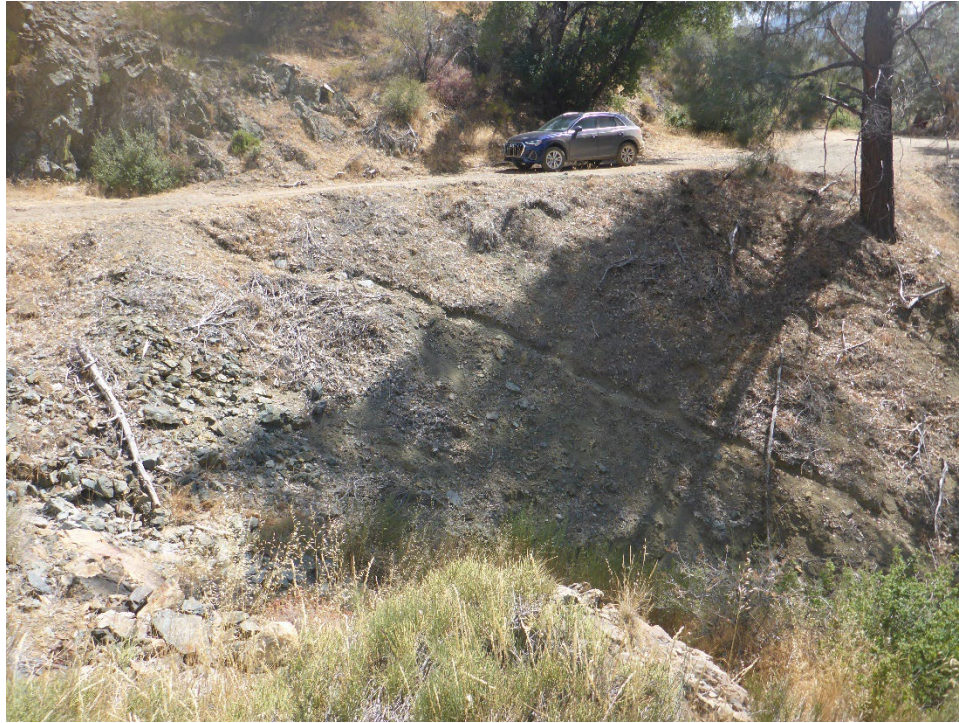
Figure A-41. Spoil material and access road at Tunnel 16/17 Spoil Site (view from immediately adjacent to right side of Figure A-40).
