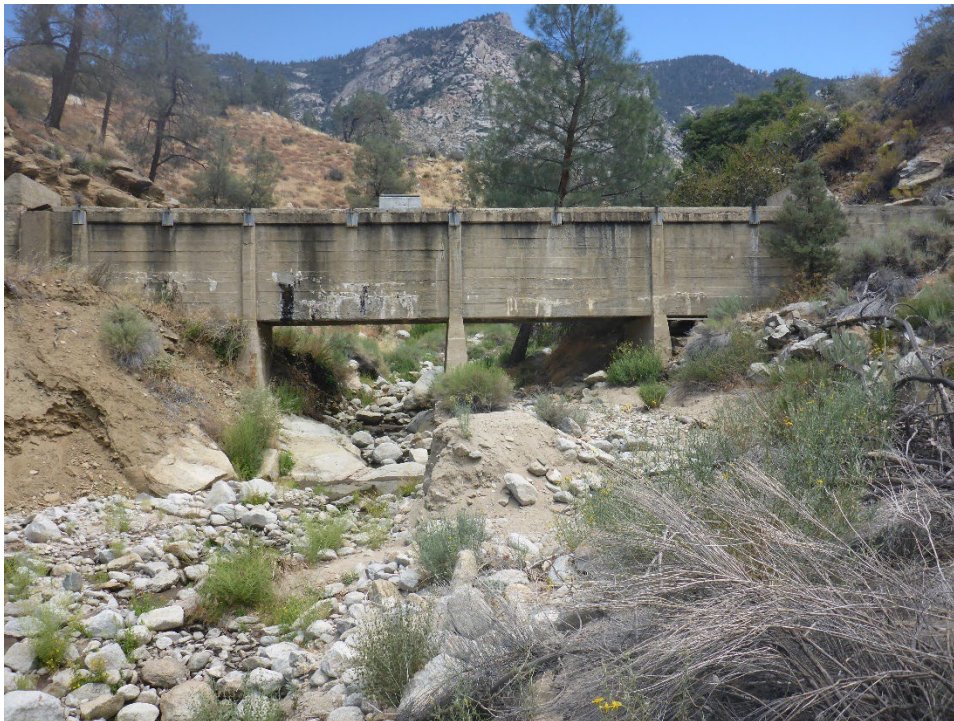
Figure A-22. Failed road crossing at Tunnel 9B/10 Spoil Site (view looking upstream from historical road–stream crossing location).
