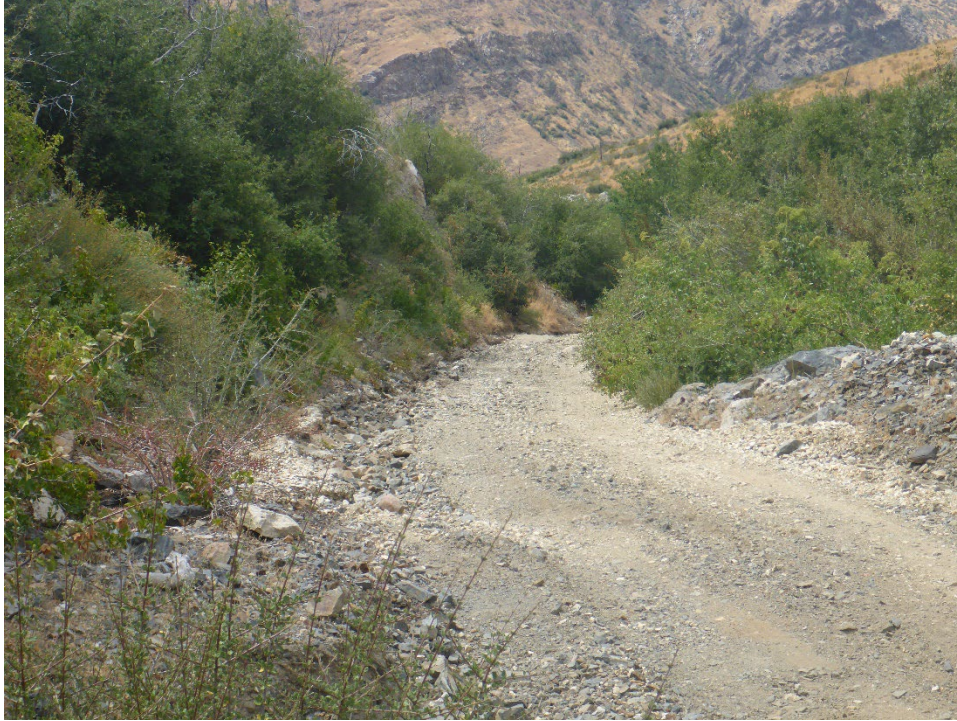
Figure A-53. Active erosion of inboard ditch along access road to Tunnel 19/20 Spoil Site.
