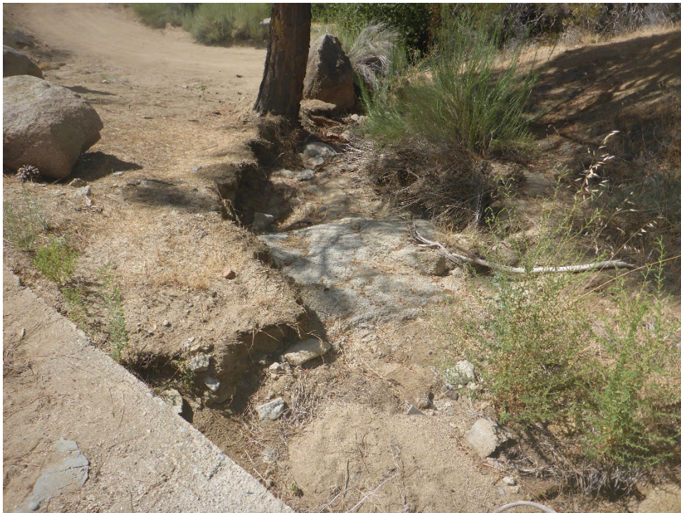
Figure A-12. Minor surface erosion at exposed tunnel section from disrupted drainage patterns.
