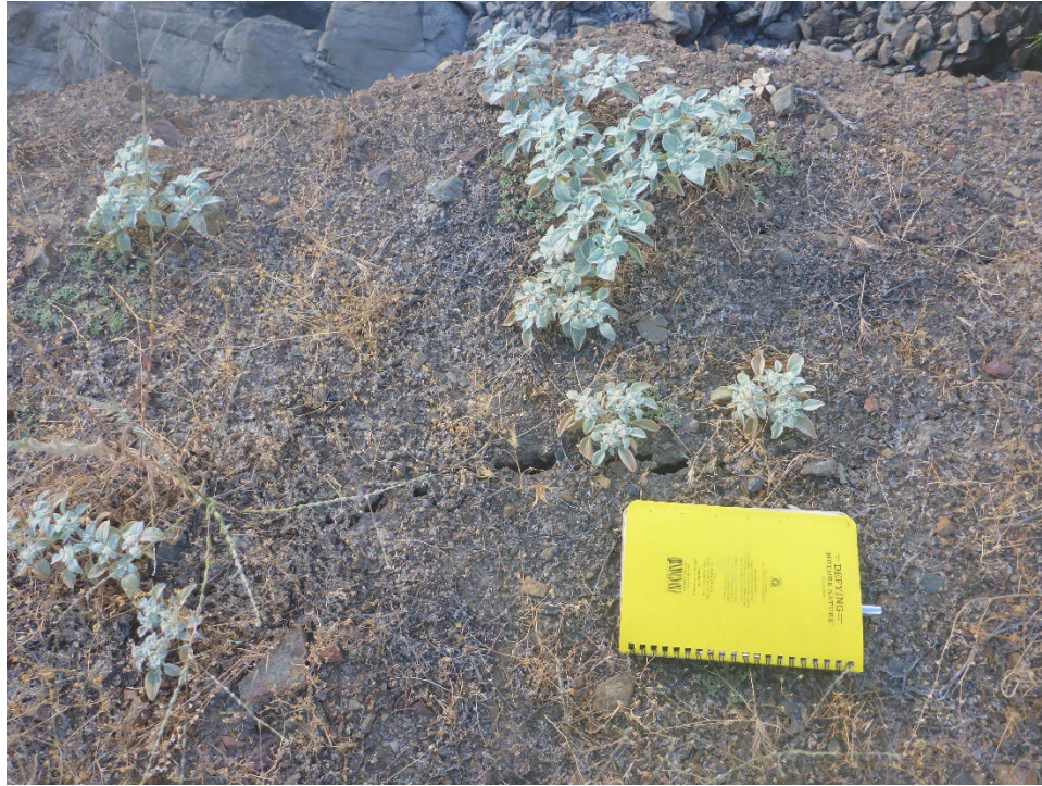
Figure A-57 Tension crack in vertical/overhanging bank of KR3 Powerhouse Forebay Spillway channel (tension crack located at the bottom edge of Figure A-57 image).
