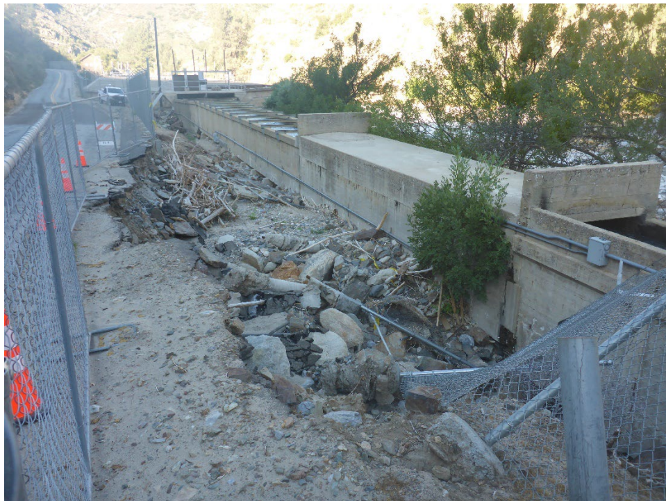
Figure A-2. Erosion of (non-Project) Mountain Highway 99 at Fairview Dam Sandbox Facility initiated by failed culvert crossing (view looking downstream).
