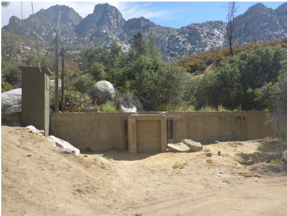
Figure A-10. Tunnel 6/7 Spoil Site showing exposed tunnel section built through drainage swale; upslope side filled to top of tunnel with sediment (view looking upslope from below tunnel).
