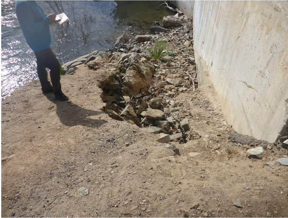
Figure A-65. Scour along base of retaining wall at KR3 Powerhouse access gate.
