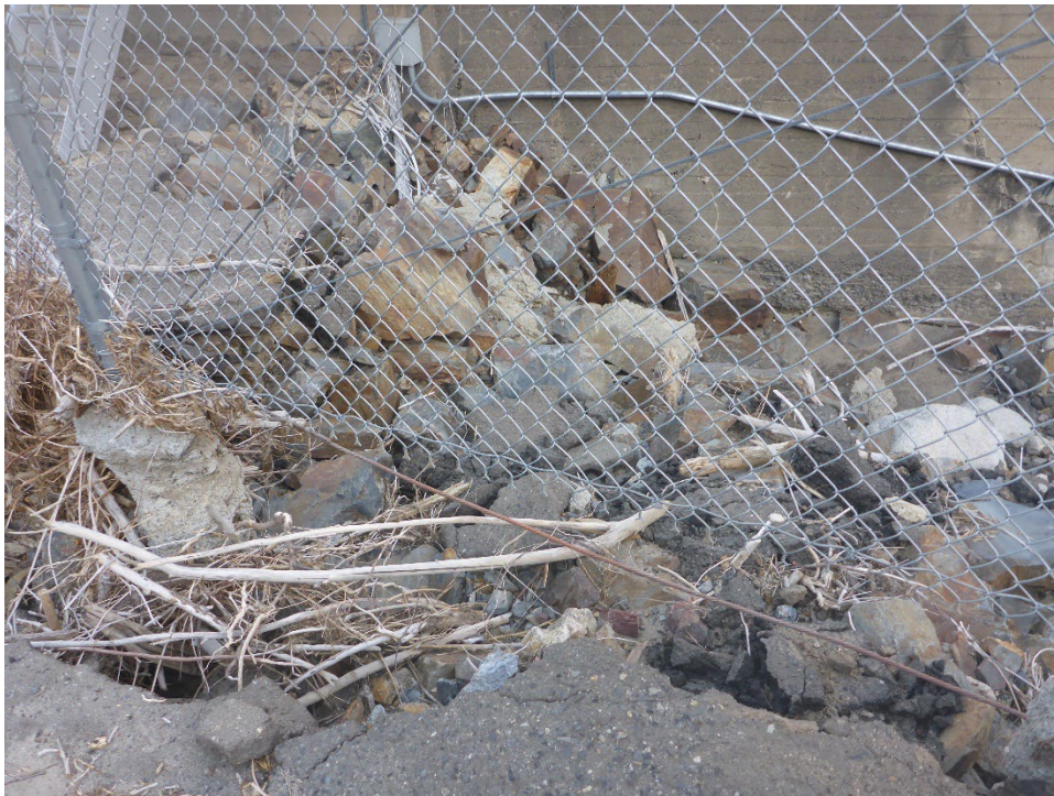
Figure A-4. Erosion and debris near access gate to Fairview Dam Sandbox Facility.
