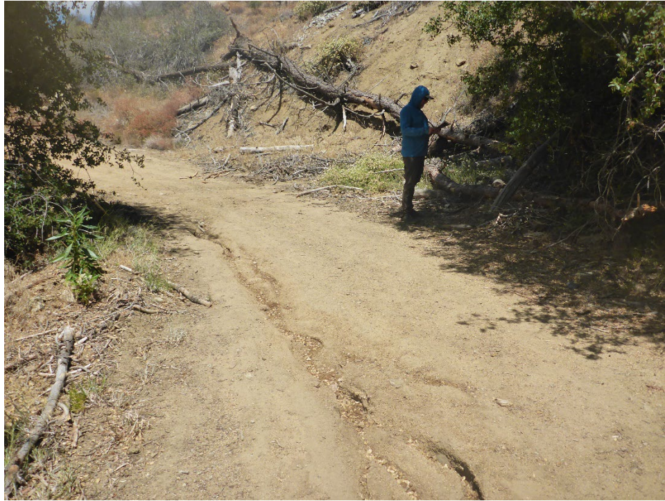
Figure A-29. Minor rilling cut into road surface at Tunnel 10 Spoil Site.
