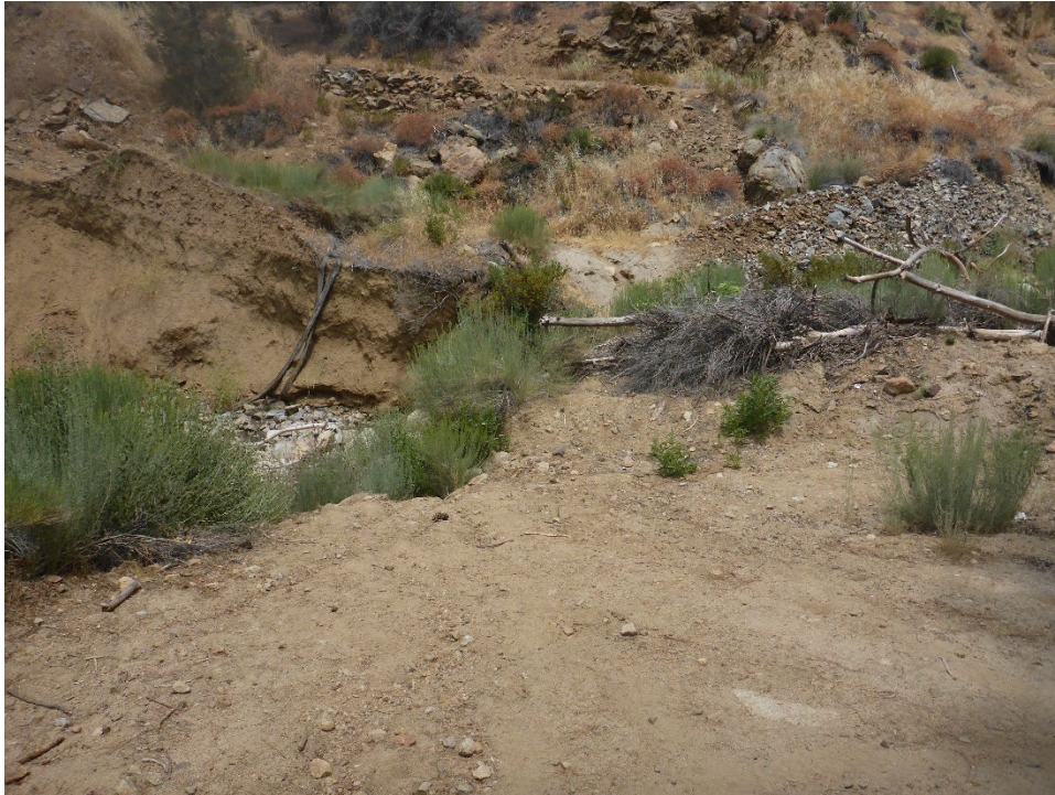
Figure A-23. Failed road crossing at Tunnel 9B/10 Spoil Site (view looking across channel at right bank [north side]).
