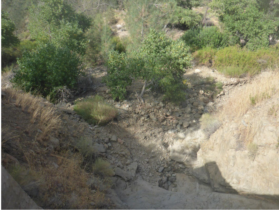
Figure A-61. KR3 Powerhouse Forebay Spillway channel where it empties into the Kern River floodplain (looking downstream).
