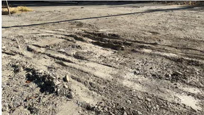
Photo D-9. August 26, 2024. Lower Powerhouse Road. Tire ruts within the lower turnout area.
