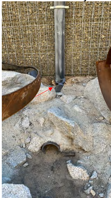
Photo D-8. August 26, 2024. Lower Powerhouse Road. Broken drainpipe (elbow; see red arrow).
