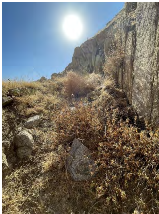
Photo D-10. August 27, 2024. Overflow Spillway Trail. Example of overgrown vegetation that is typical of this trail.
