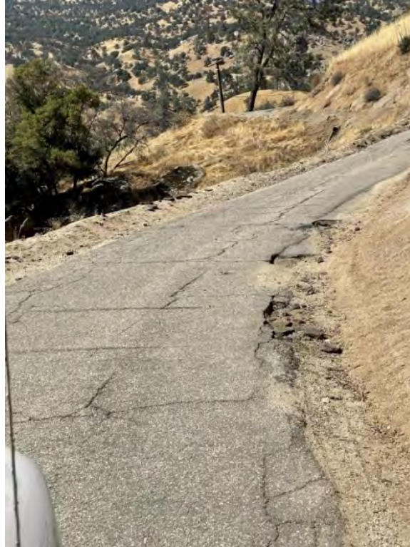
Photo D-3. August 26, 2024. Democrat Dam Road. Example of road surface erosion present throughout this road.
