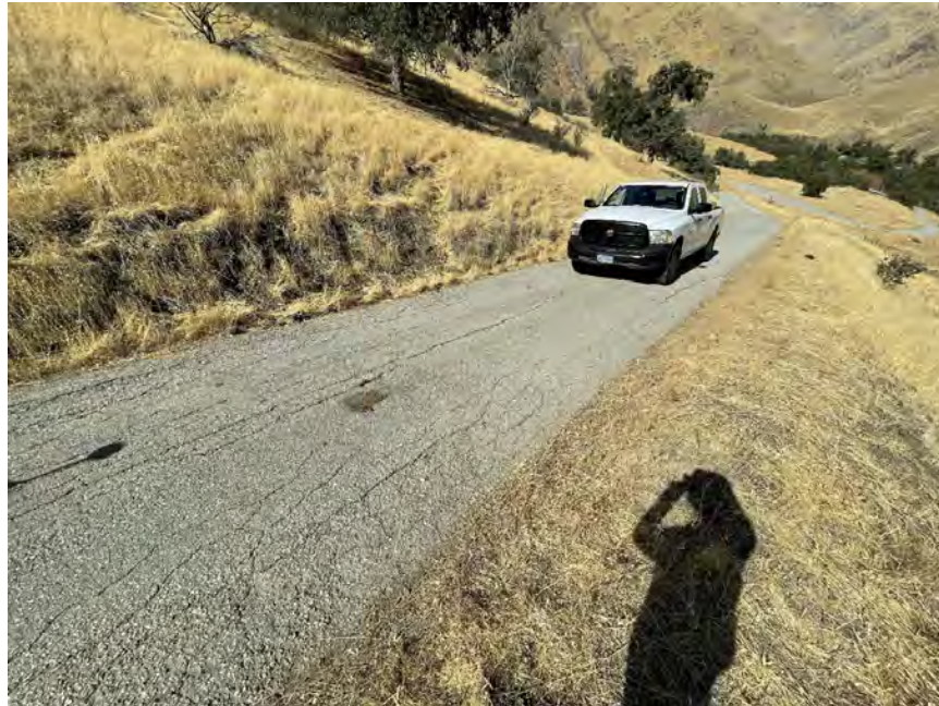
Photo D-13. August 26, 2024. Stark Creek Road. Low to moderate cracking along approximately 150 feet of roadway.
