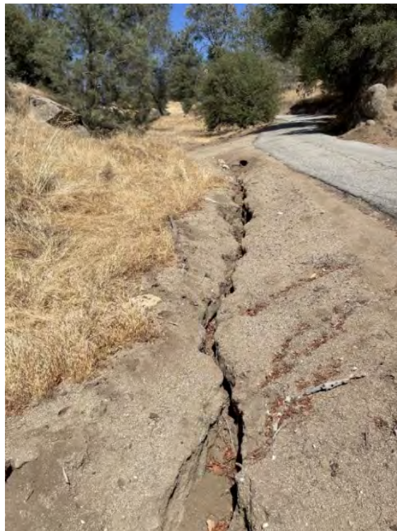
Photo D-4. August 26, 2024. Democrat Dam Road. Gullying present along several hundred feet of roadway below culvert.
