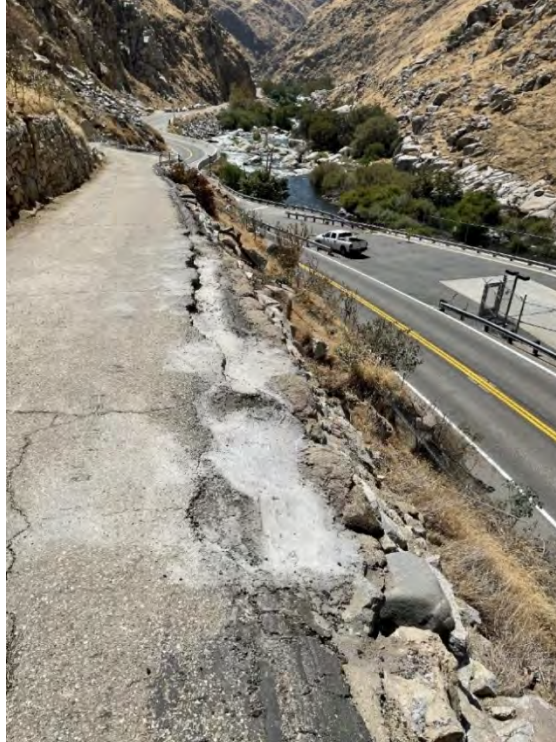
Photo D-7. August 27, 2024. Forebay Operations Area Road. Gap in curb along approximately 20-25 feet of roadway.
