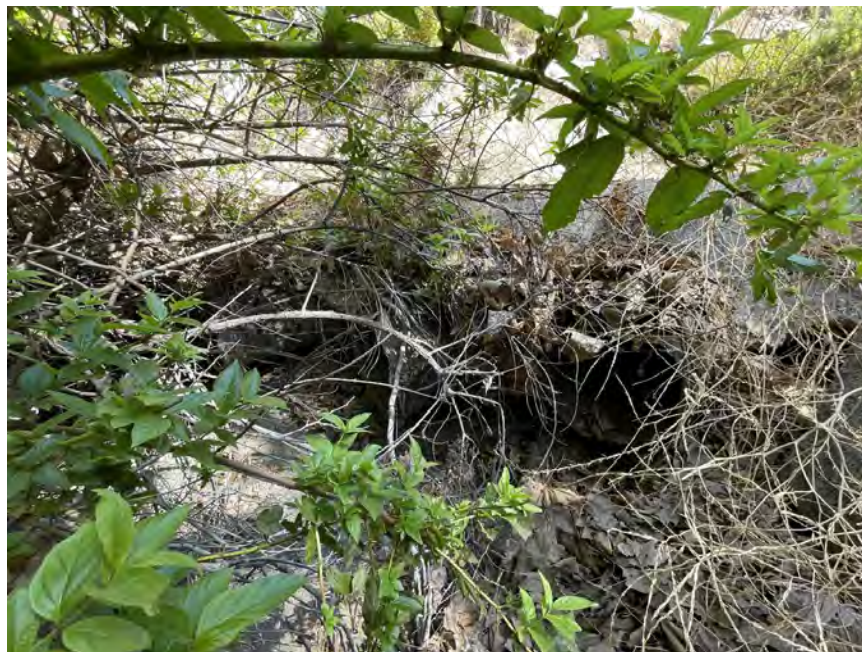
Photo D-14. August 26, 2024. Stark Creek Road. Upstream side of low-water crossing along Stark Creek. Accumulated vegetative debris obscured the CMP underneath the cement slab, but the easternmost CMP appeared to be crushed.
