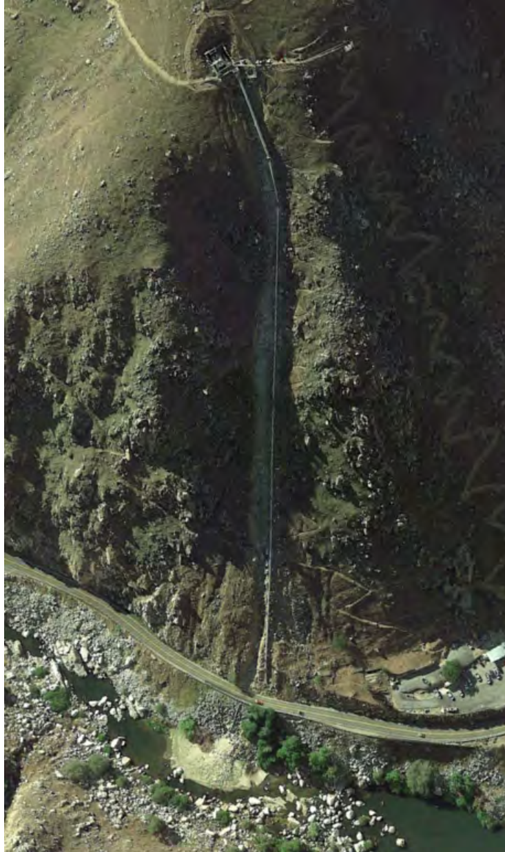
Photo A-22. KR1 Penstock Erosion and Sediment Deposition in the Kern River Channel After the August 20, 2013, Forebay Spill Event (Google Earth Image, Date: 4/15/2014)
