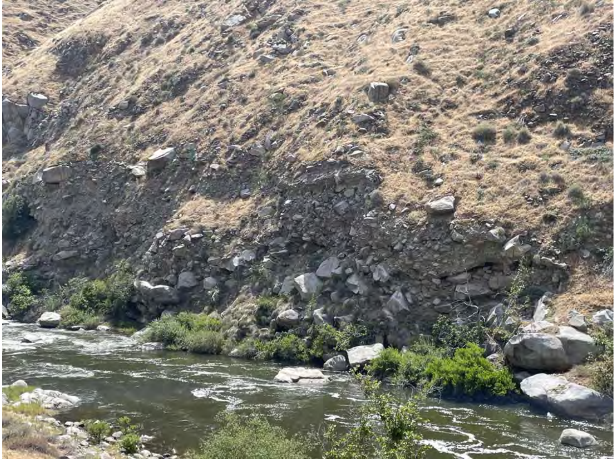
Photo A-16. Bank Erosion RB-2
