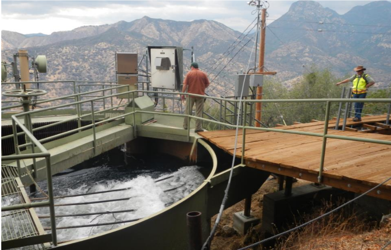
Figure AQ 9-5. Kaweah No. 1 Forebay Tank.
