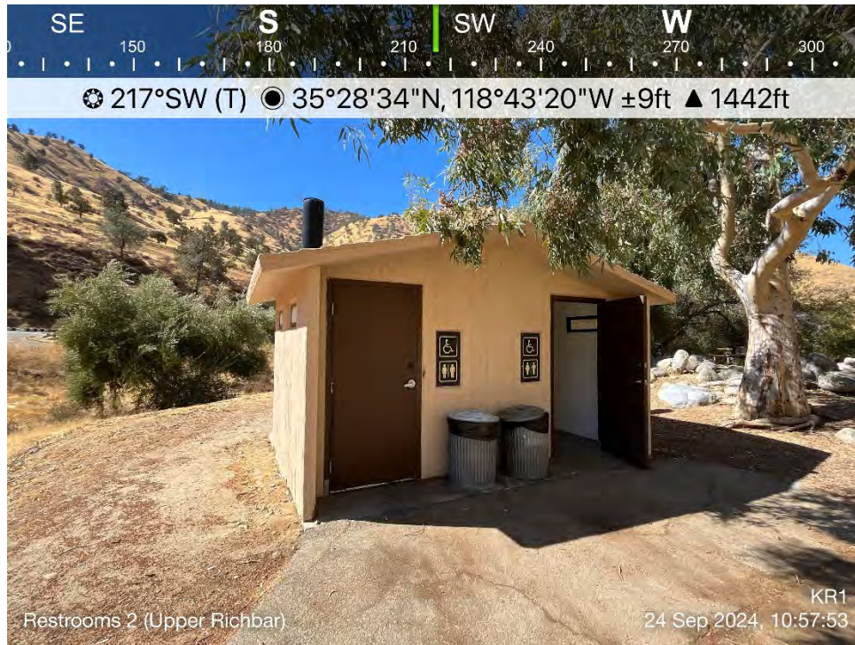
Photo B-32. Upper Richbar Day Use Area – Pit Toilets #2
