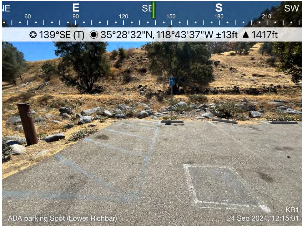
Photo B-54. Lower Richbar Day Use Area – ADA Parking Spots
