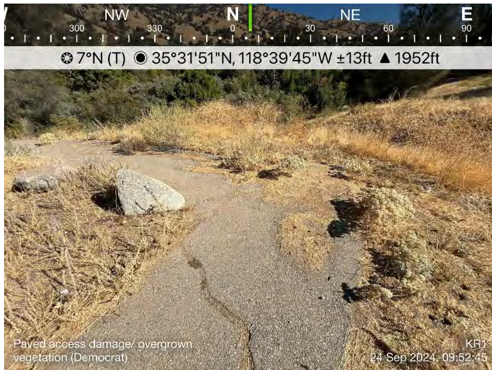
Photo B-11. Democrat Raft Take-out Boating Site – Paved Access Path and Overgrown Vegetation
