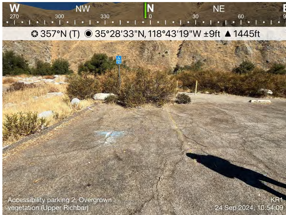
Photo B-27. Upper Richbar Day Use Area – East Parking Lot and ADA Parking Spots
