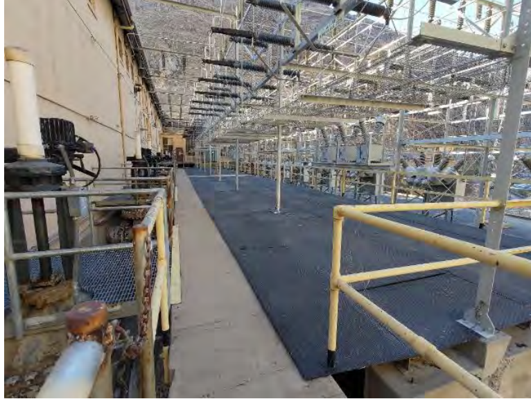
Photo G-31. Kern River No. 1 Switchyard: The facility consists of active electrical equipment and potential roosting areas are highly exposed to the elements or electrical current. Facility is not suitable for roosting but bats may pass through to enter the Powerhouse.
