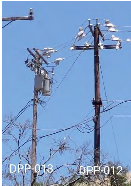
DPP-13. Configuration 11: Three-Phase Transformer Bank
