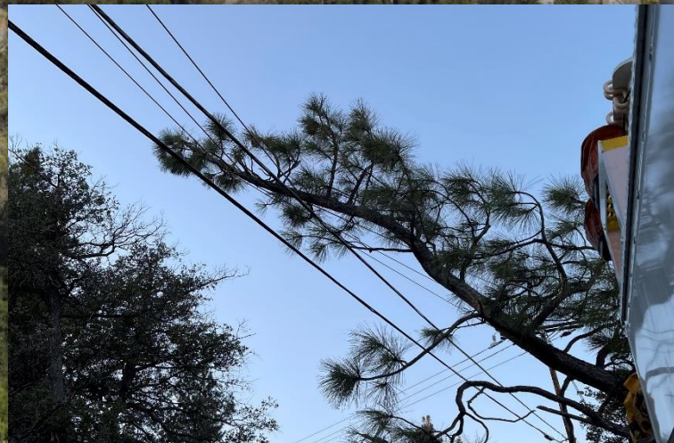
Damage/hazards found after strong winds during PSPS
