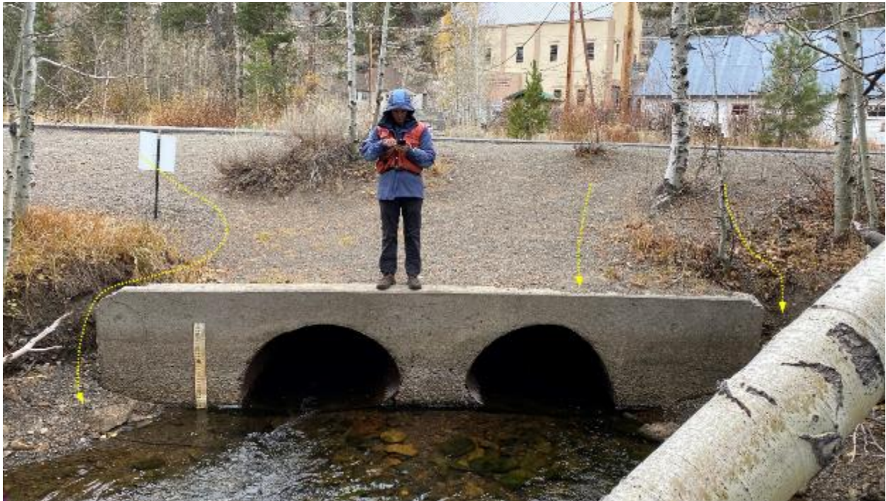
Photo AQ 5-30. Surface and bank erosion at the outlet side of the tailrace SR-158 culvert (location RE-4).
