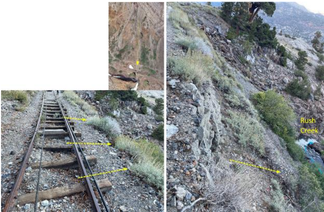
Photo AQ 5-52. Surface erosion from around the tramway (lower left) and hillslope erosion below the retaining wall (right) from a combination of prior tram/wall construction/repairs and mass wasting of the mountainside (top left). Location PE-10.
