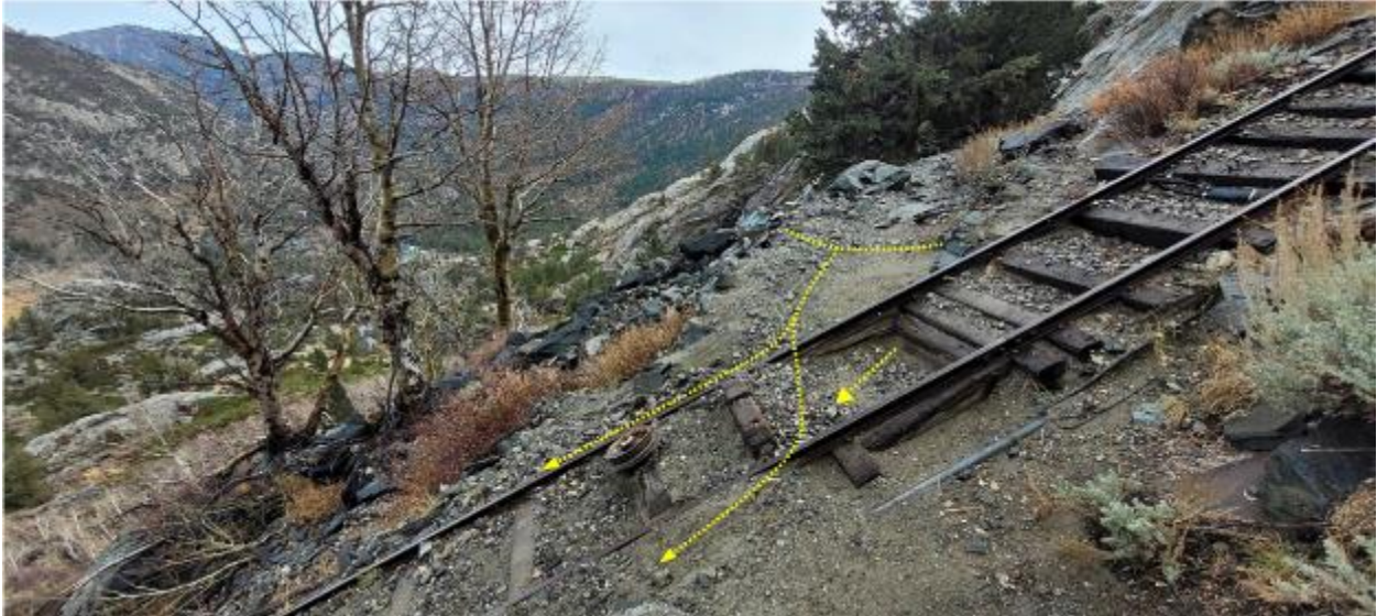
Photo AQ 5-25. Example of worn concave trail surface and erosion at the intersection of the tramway (location TE-3).
