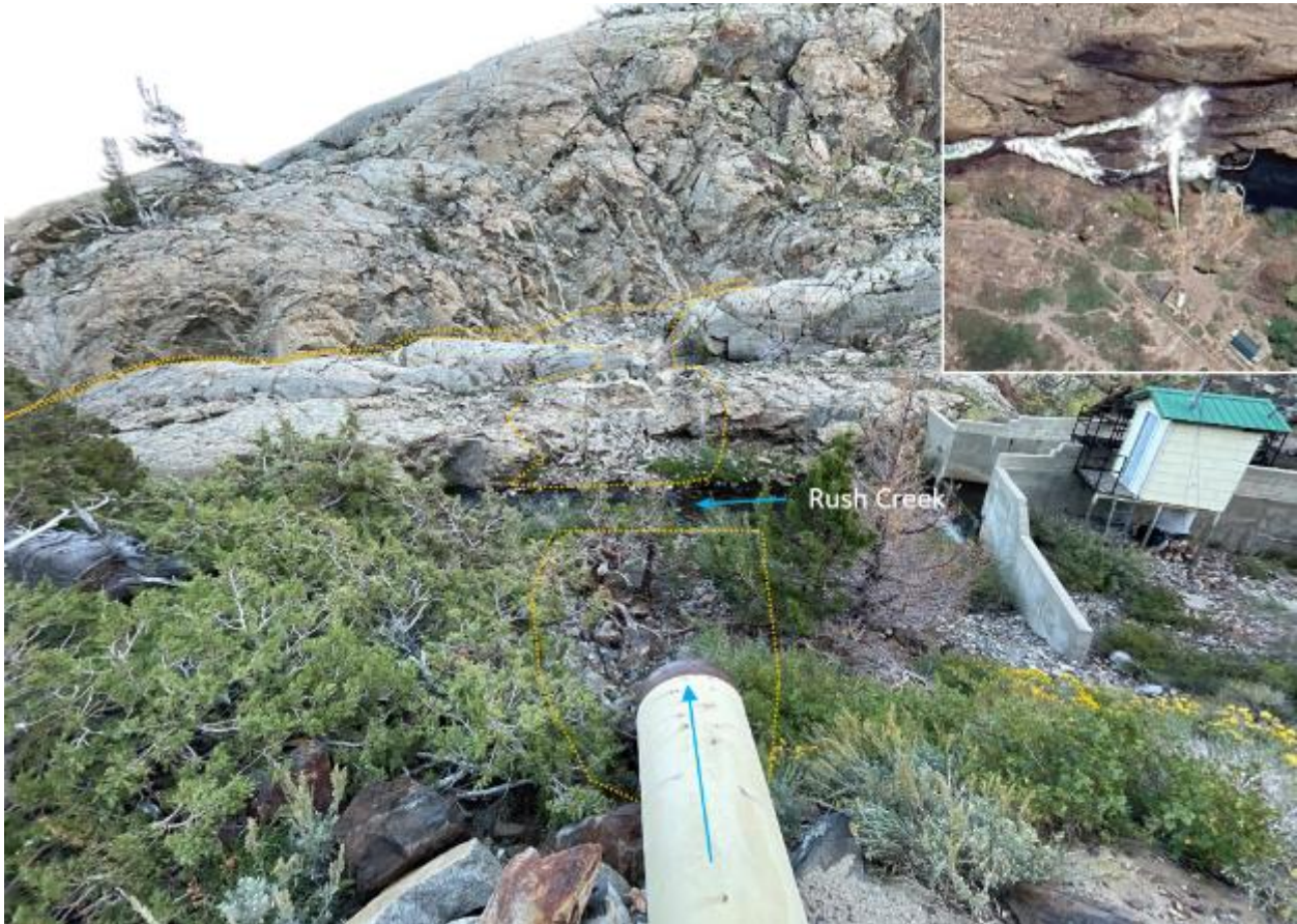
Photo AQ 5-50. Agnew junction valve house 18-inch standpipe outlet and the area eroded on the right and left bank of Rush Creek (location PE-8).
