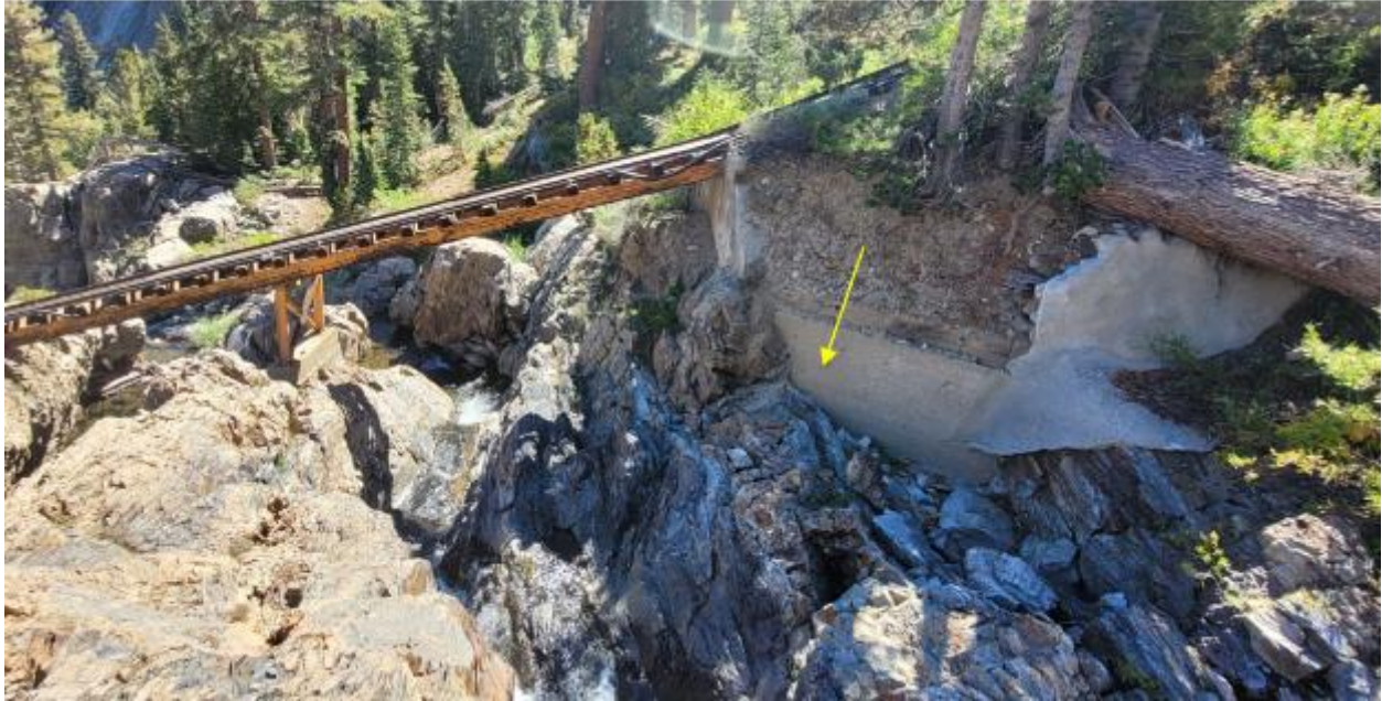
Photo AQ 5-45. Erosion of the right bank side of the tram bridge abutment retaining wall (location PE-4).
