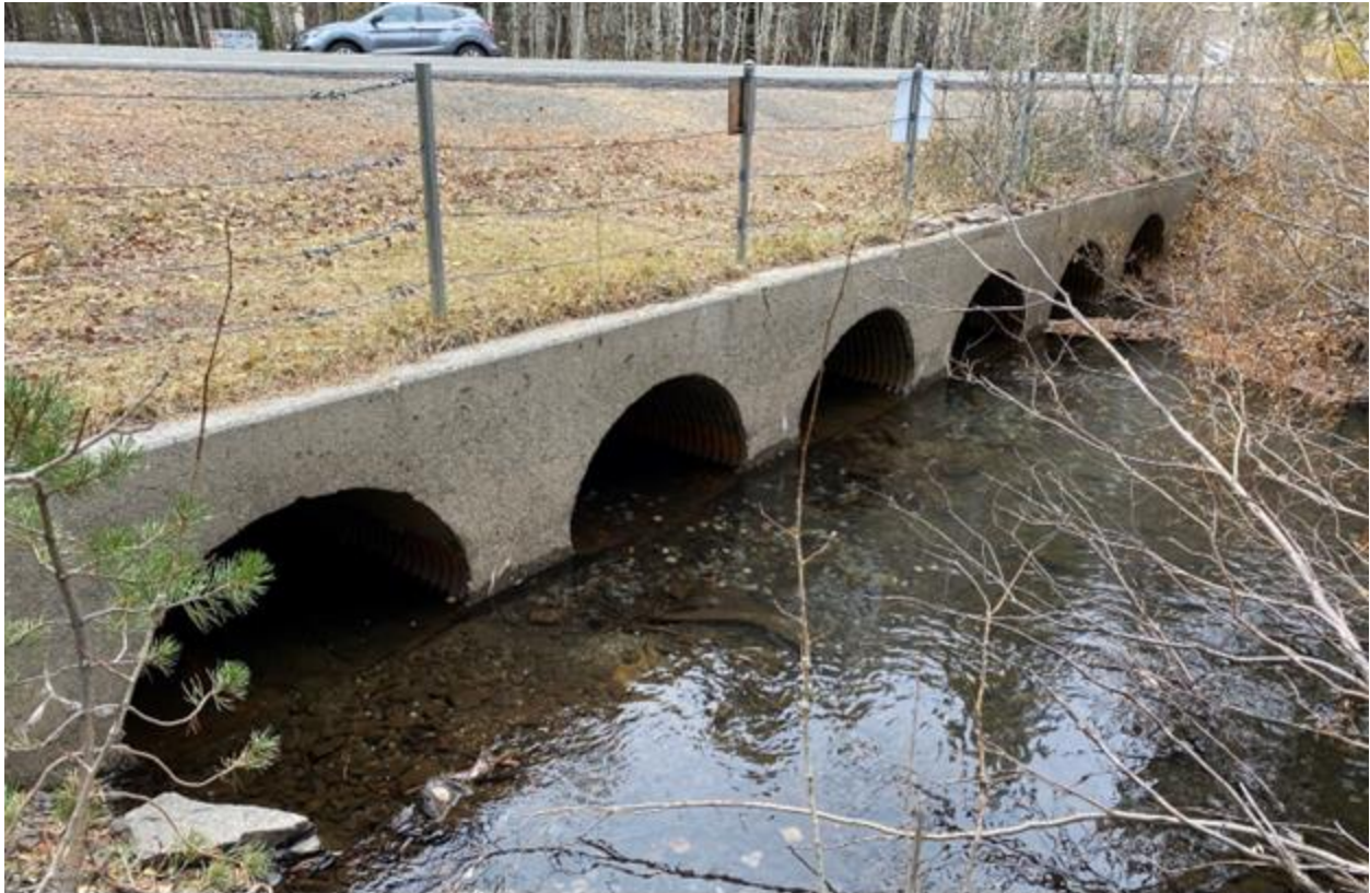
Photo AQ 5-31. Minor surface erosion from the shoulder/turnout at the outlet side of the Rush Creek SR-158 culverts (location RE-5).
