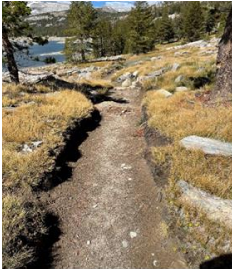
Photo AQ 5-23. Prolonged surface wear and erosion of the trail bed coupled with diversion of surface flow from upslope has caused incision (location TE-1).
