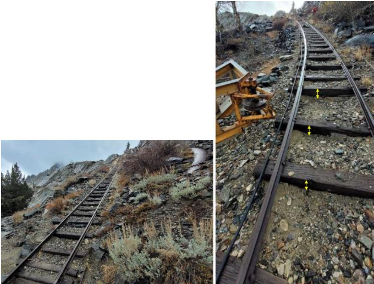
Photo AQ 5-53. Typical surface erosion from around the rail ties in the middle portion of the tramway below Agnew (location PE-11).
