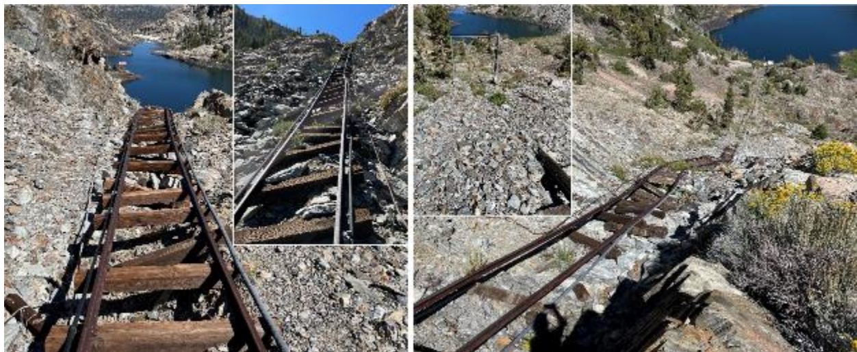
Photo AQ 5-48. Various perspectives of the eroded tramway caused by runoff diversion from the culvert crossing that became plugged in the 2017 runoff season (location PE-6).
