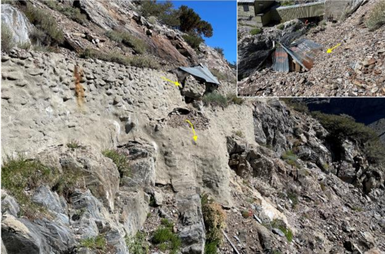
Photo AQ 5-43. Rock and shotcrete/gunite retaining wall failures below the Gem to Agnew junction flowline and slumping/collapsing in around the shack (upper right photo). Location PE-2.
