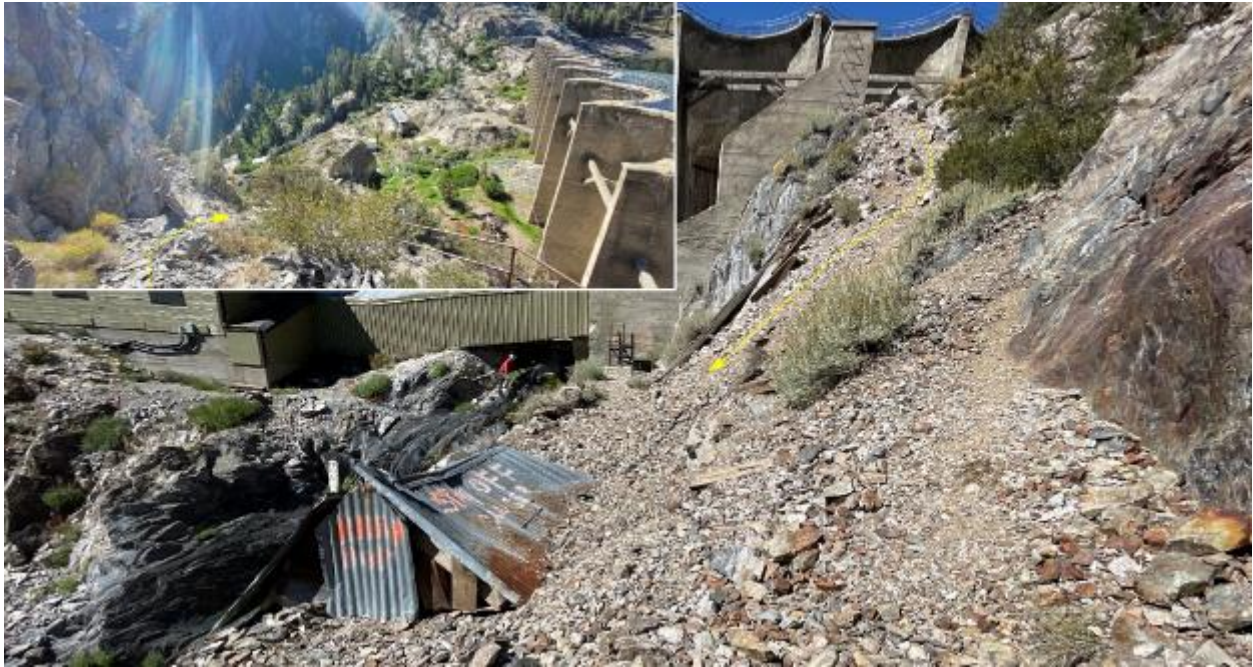
Photo AQ 5-27. Surface erosion from the Lower Gem Dam Trail (location TE-5).
