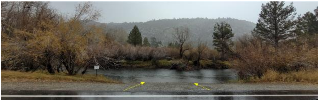
Photo AQ 5-28. Sheet/bank erosion along SR-158 turnout and stream access (location RE-1).
