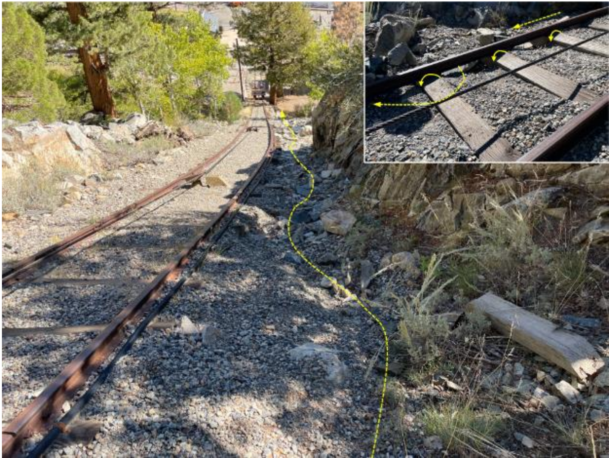
Photo AQ 5-55. Typical surface erosion along steeper pitches of the lower Agnew tramway (note the gap beneath the rail and rotated tie). Rill erosion along the lower side of the tracks leading towards the powerhouse (location PE-13).
