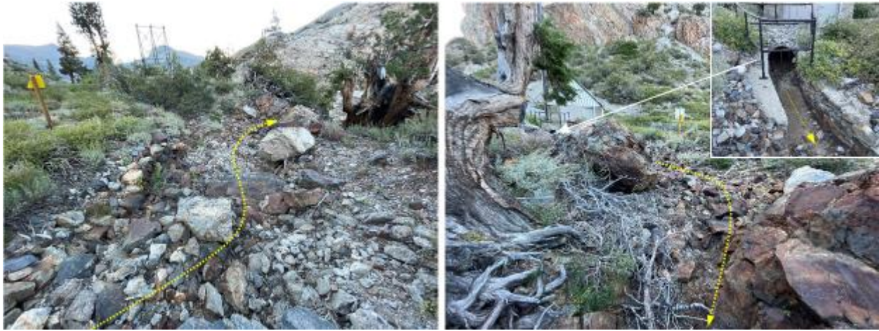
Photo AQ 5-51. Erosion of a channel below the Agnew junction valve house to Rush Creek (location PE-9).
