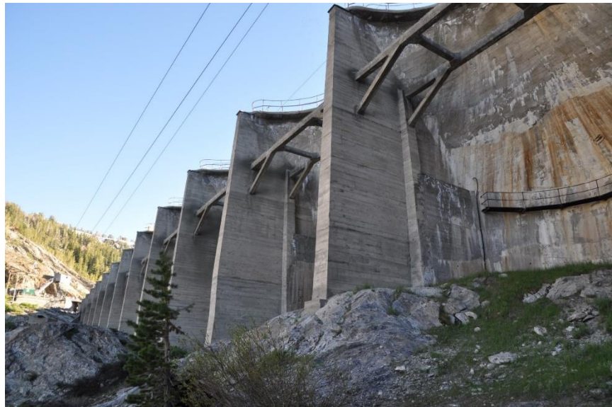
Photo 2. Gem Dam. This facility was determined to be suitable bat roosting habitat. The dam contains cracks in concrete overhangs and has appropriate thermal conditions (high solar exposure).
