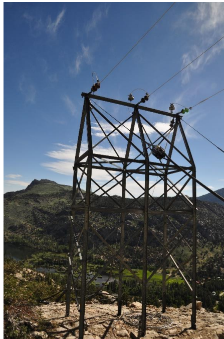
4423283E. This photograph shows a tower with jumper wires that are assumed to be uninsulated. This tower poses a potential risk for avian electrocution.
