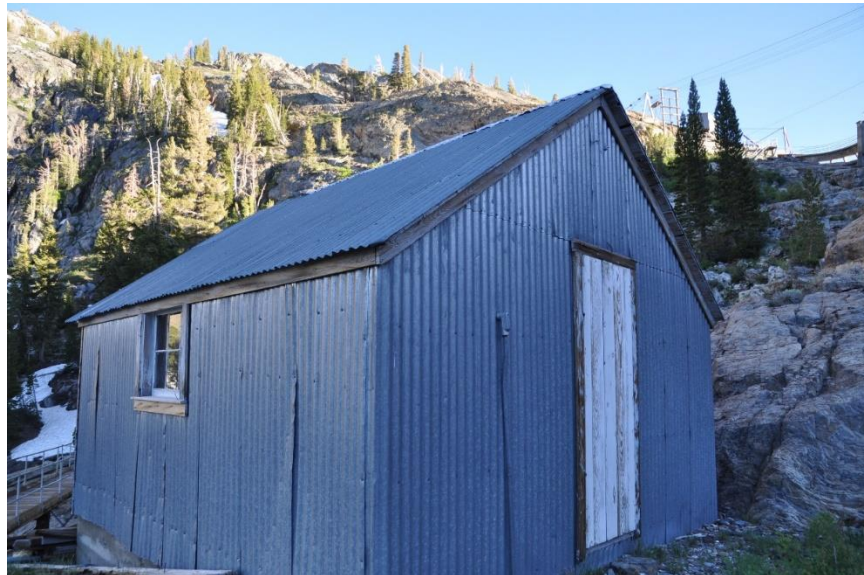
Photo 20. Gem Cookhouse. This facility was determined to be suitable bat roosting habitat. This building contains suitable roofed elements for bat roosting, and has a broken window and gaps in the metal siding for bats to enter. The roof is a corrugated metal sheet with enough spacing for bats to roost under the eaves. Building is located in an area that has appropriate thermal conditions for maternity roosting (high solar exposure).
