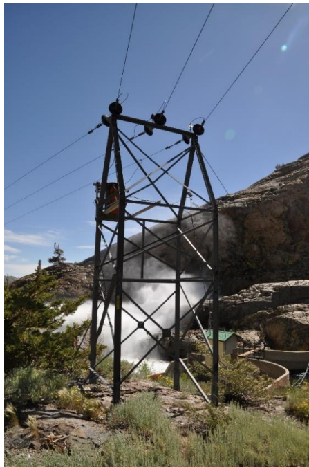
4423287E. This photograph shows a tower with one transformer. This tower design poses a potential risk for avian electrocution.
