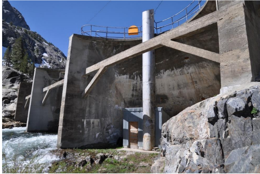
Photo 9. Agnew Dam Valve House. This facility was determined to be suitable bat roosting habitat. Crack above door provides access; corrugated metal roof provides suitable roofed element. Because of the proximity to dam outlet pipes and shady position, building is likely colder than surrounding conditions. Cold buildings are not preferred for maternity roosting, but could be used for hibernation.
