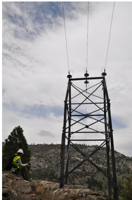
4423279E. This photograph shows a tower that has uninsulated jumper wires and uninsulated phase conductors that are less than 60 inches apart. This tower design poses a potential risk for avian electrocution.
