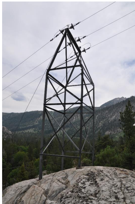
4840586E. This photograph shows a tower that has uninsulated jumper wires and uninsulated phase conductors that are less than 60 inches apart. This tower design poses a potential risk for avian electrocution.
