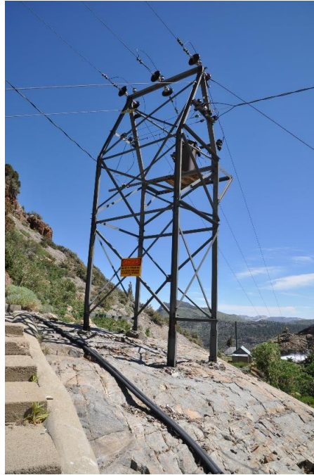
4423288E. This photograph shows a tower with one transformer. This tower design poses a potential risk for avian electrocution.
