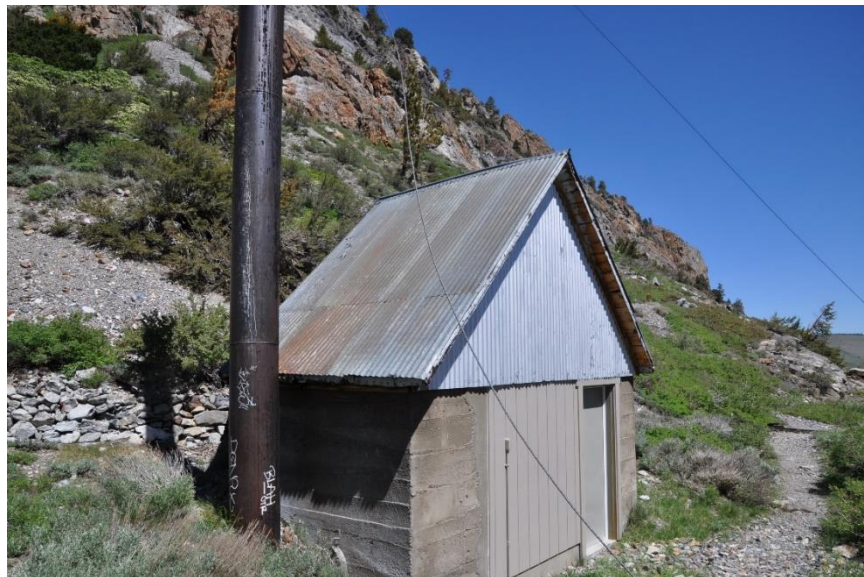
Photo 8. Agnew Junction (Valve House and Stand Pipe). This facility was determined to be suitable bat roosting habitat. Building contains overhangs with cracks along the corrugated metal roof that could provide access to interior.
