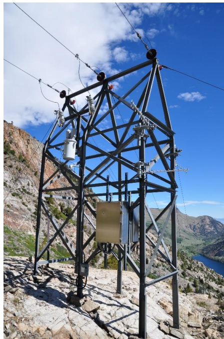
4423285E. This photograph shows a tower with a transformer and uninsulated jumper wires and guy wires. This tower poses a potential risk for avian electrocution.
