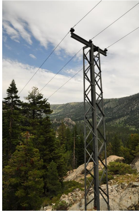
4423280E. This photograph shows a tower with uncovered phase conductors that are less than 60 inches apart. This tower design poses a potential risk for avian electrocution.
