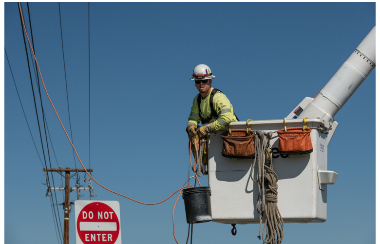
An SCE lineman works on a covered conductor installation, a critical wildfire mitigation tool.
