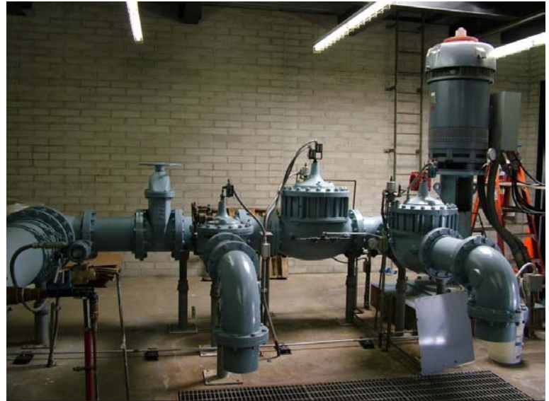
Motors drive a water pump for one of the City of Downey's groundwater wells. The City is saving energy and money by working with SCE to replace motors and pumps through the Agricultural Energy Efficiency Program.
