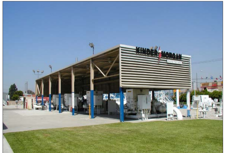
Pipeline transportation and energy storage firm Kinder Morgan participates in SCE energy efficiency and demand response programs to save on power costs at its Southern California facilities, including the Watson pump station in Carson.
