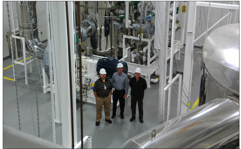
The estimated annual electricity savings for B. Braun's new Water for Injection (WFI) system (to manufacture purified water for IV solutions) total nearly 3.3 million kilowatt-hours. Shown on-site are (left to right) company officials Nima Bayan, Ron Danfield and Bob Panza.
