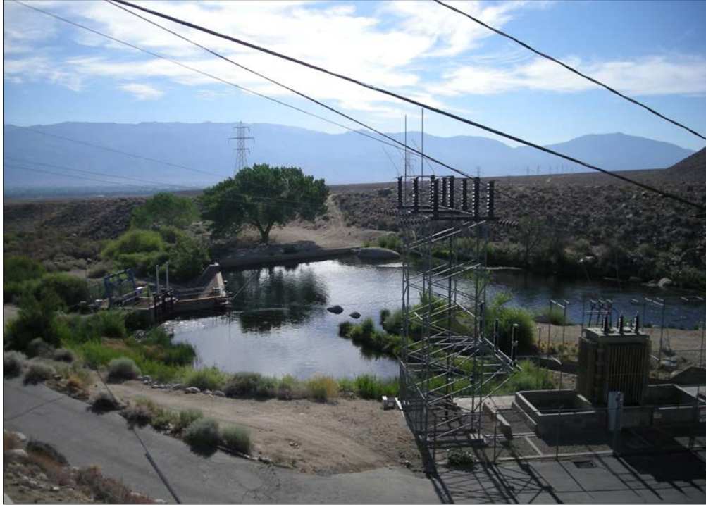
Photo 9.10-5. Plant No. 5 Facilities
