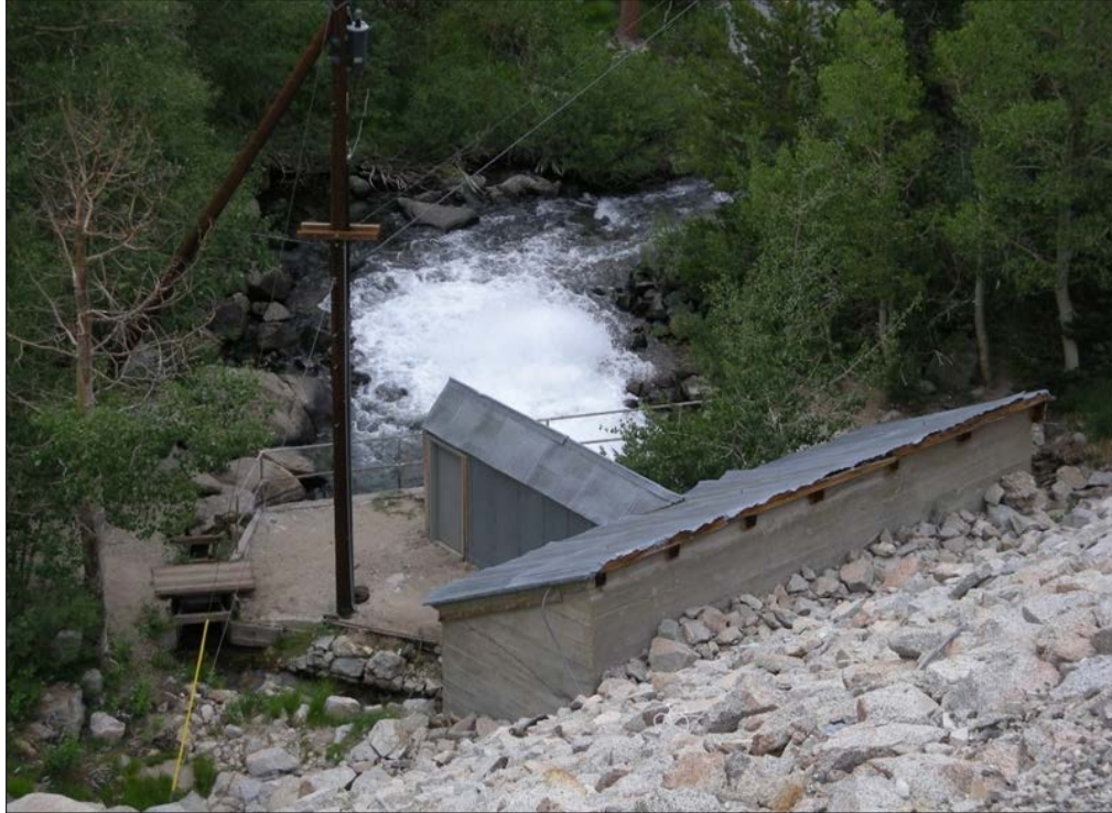
Photo 8.10-21. Lake Sabrina Low Level Outlet Release to Middle Fork Bishop Creek.
