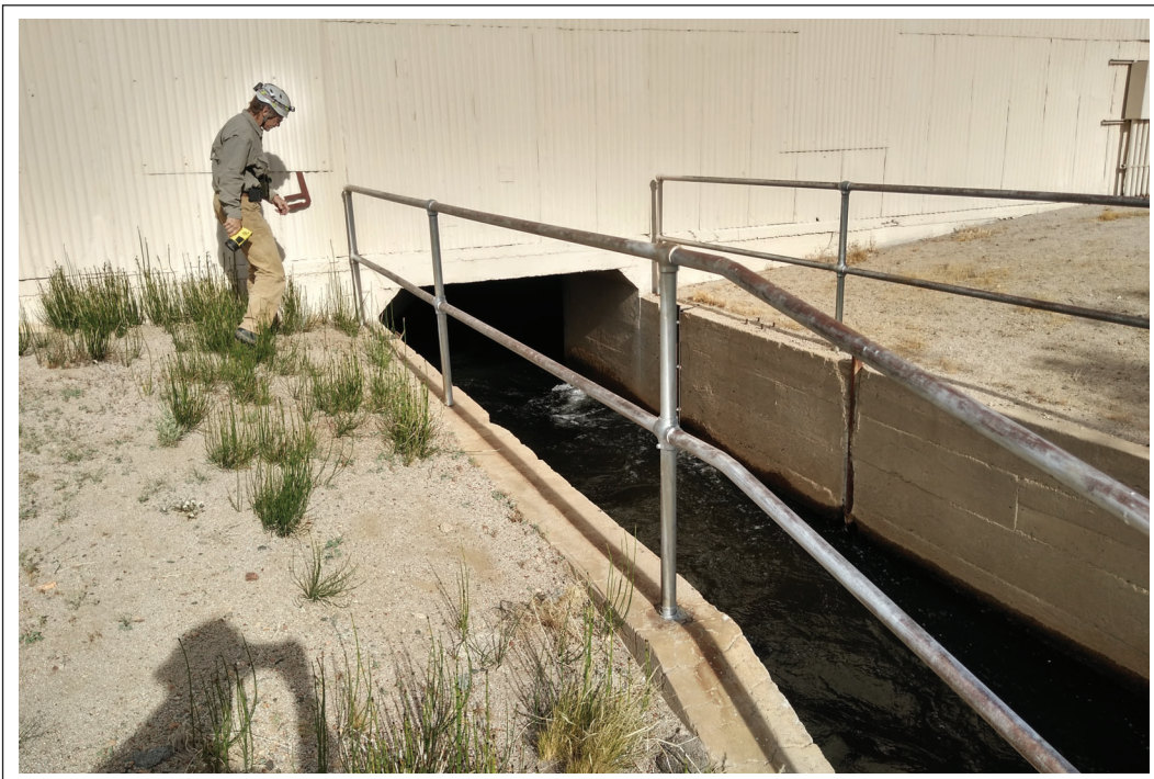
Powerhouse No. 5: View of the tailrace facing west. This larger tailrace does not completely inundate during facility flushing events leaving potentially suitable bat roosting habitat.
