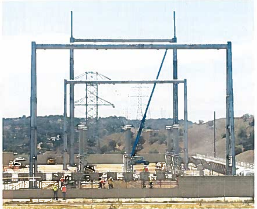
Western Transition Station.
