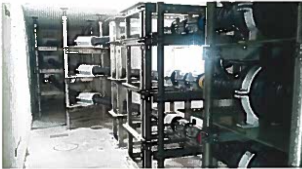
Underground cable racking.
