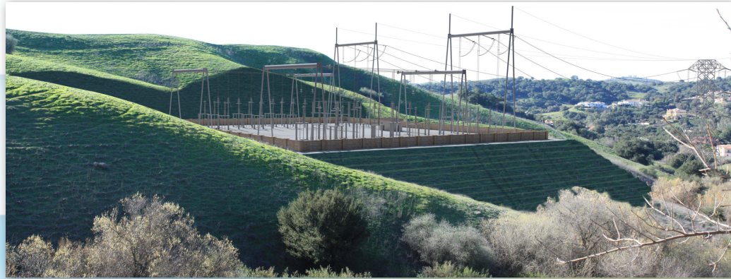
Simulated view looking southwest from the hillside behind the row of homes on the south side of Avenida Compadres toward the WTS.
