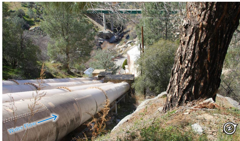
Figure 2-55. Penstocks (Photo Date: 03/2022)
