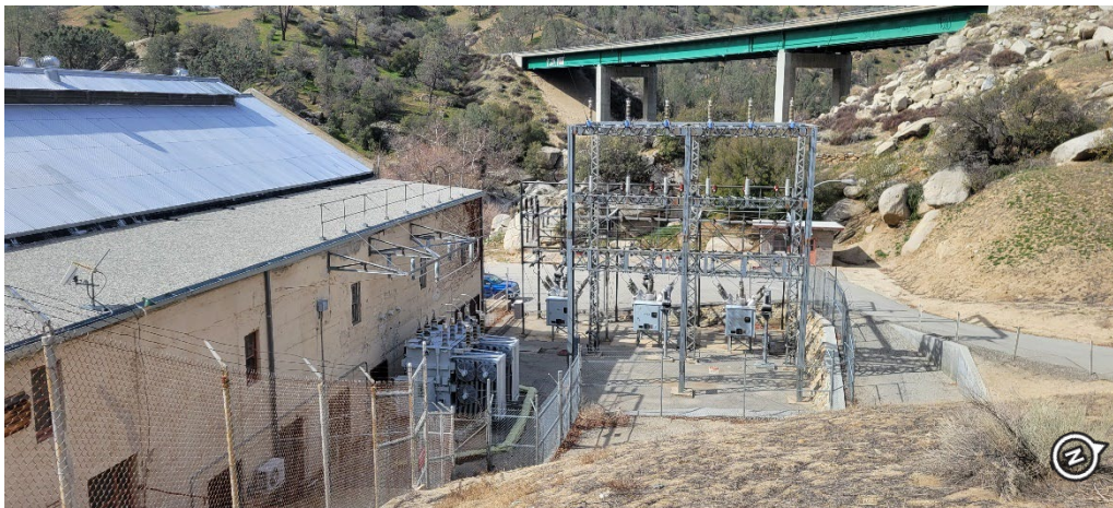
Figure 2-60. Borel Switchyard and Powerhouse (Photo Date: 03/2022)
