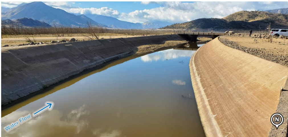
Figure 2-8. Concrete-lined Canal and Bridge, Looking Downstream (Downstream of Tilley No. 1 Concrete Flume) (Photo Date: 02/2021)
