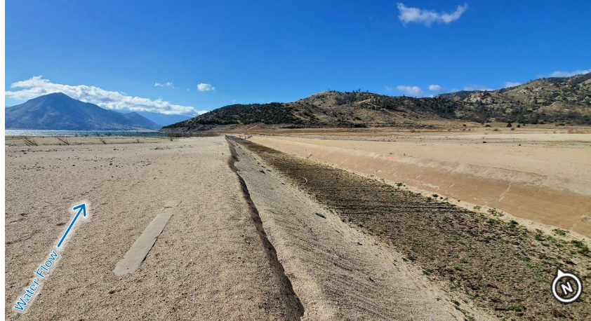
Figure 2-12. Concrete-lined Canal Downstream of Tilley No. 3 Concrete Flume, Looking Downstream (Photo Date: 02/2021)
