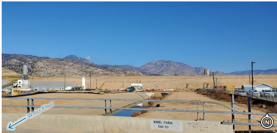
Figure 2-25. Federal Lands Administered by the Corps with Filled Canal and Auxiliary Dam, Looking Upstream (Photo Date: 01/2020)
