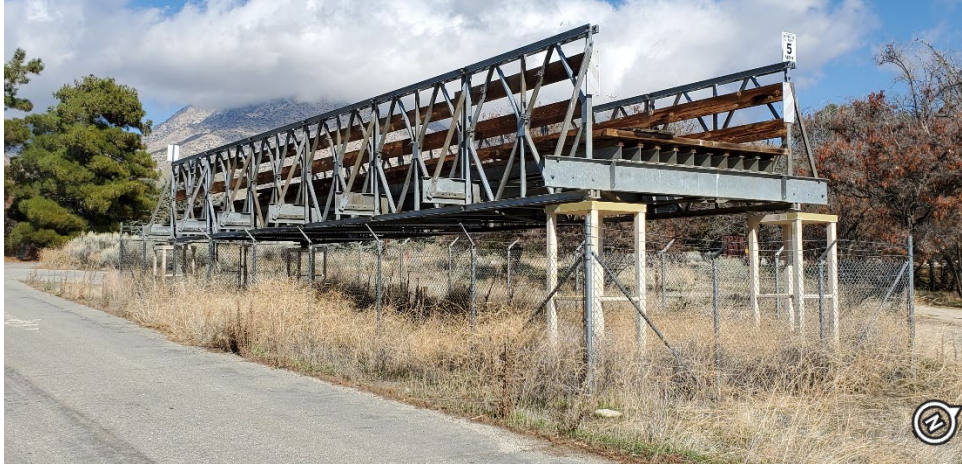
Figure 2-16. Bailey Bridge, Stored on Federal Lands Administered by the Forest Service (Photo Date: 02/2021)
