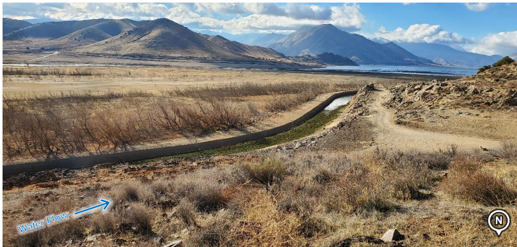
Figure 2-5. Canal from Canal Inlet Structure to Tilley No. 1 Concrete Flume (out of frame)(looking downstream). (Photo Date: 02/2021)
