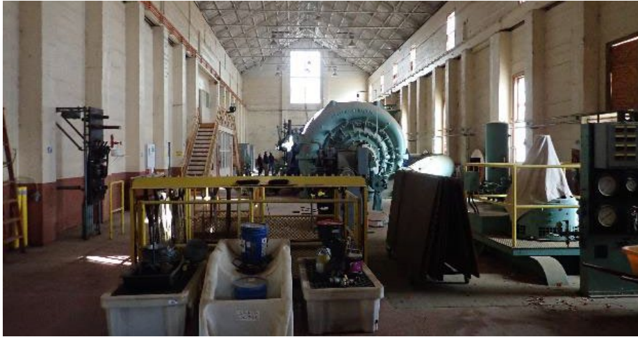
Figure 2-56. Powerhouse Interior (Photo Date: 01/2020)
