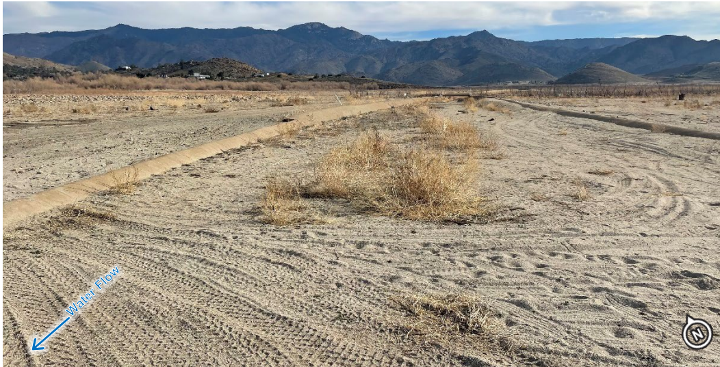
Figure 2-9. Canal Filled with Sedimentation, Looking Upstream (Downstream of Tilley No. 2 Concrete Flume) (Photo Date: 03/2022)
