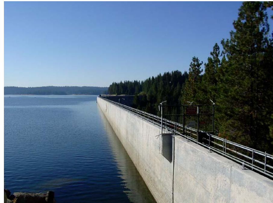
KOP 15 - Photo 15b View of Shaver Lake Dam looking south from Shaver dam turnout (October 3, 2001)
