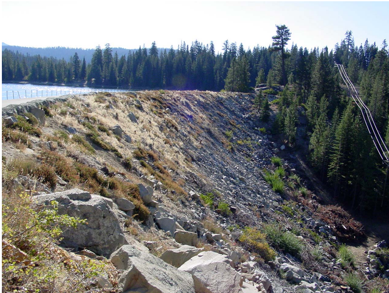
K0P 6 - Photo 6a View of Huntington Lake looking south from Dam 3 (October 1, 2001)
