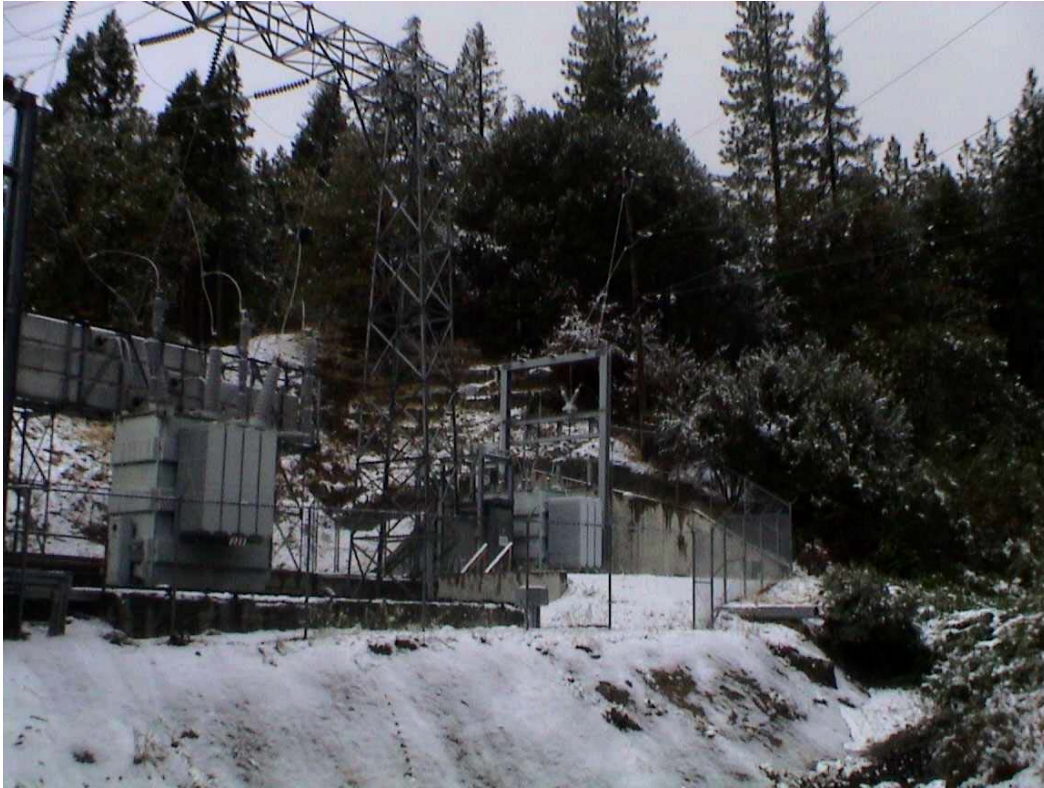
Photo C-5 – Powerhouse No. 1 Switchyard. This photograph shows the clearing of brush and woody debris around the perimeter of the facility.
