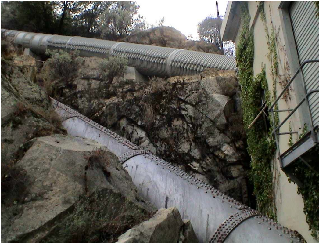
Photo C-15 - Powerhouse No. 8. This photograph shows the steep rock hillside behind Powerhouse No. 8. This hillside has little vegetative cover and provides a defensible space around the structure.
