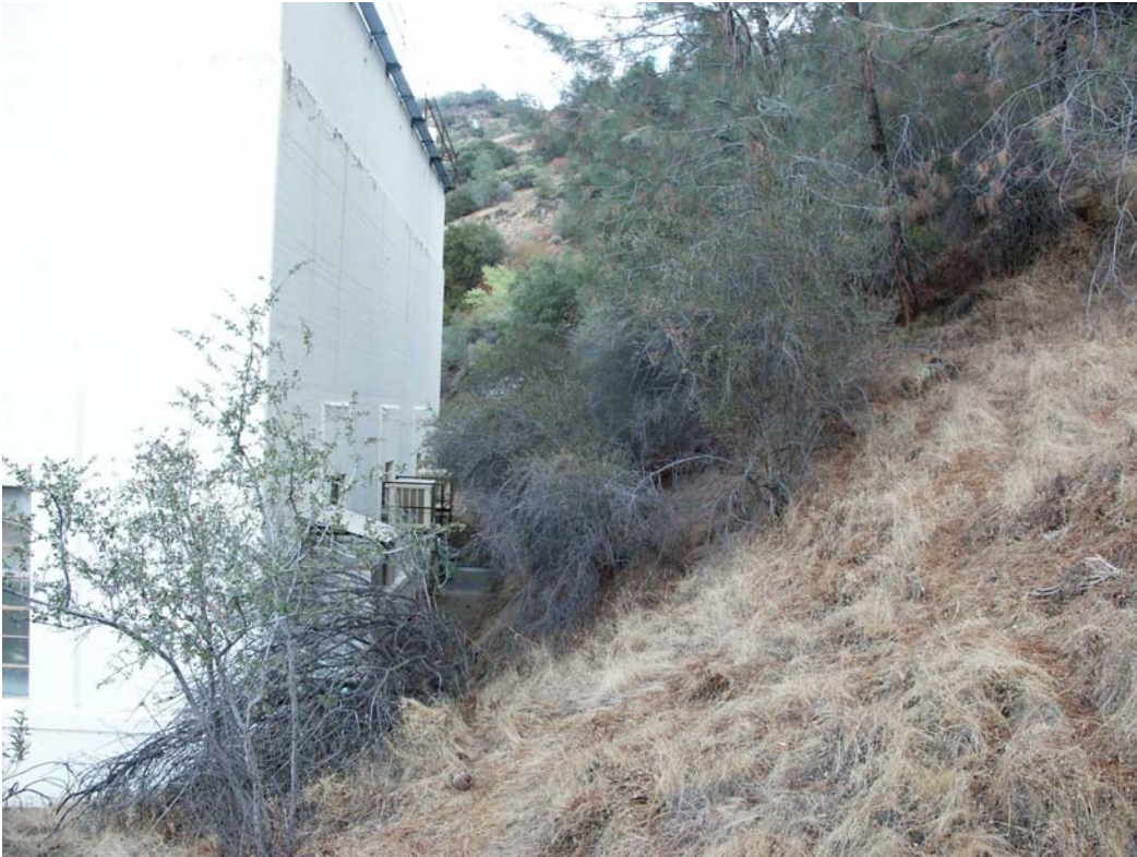
Photo C-21 – Powerhouse No. 3. This photograph shows brush encroaching behind the powerhouse building. The vegetation could be cleared back to provide a better defensible space. The building is of concrete construction which provides good fire protection.
