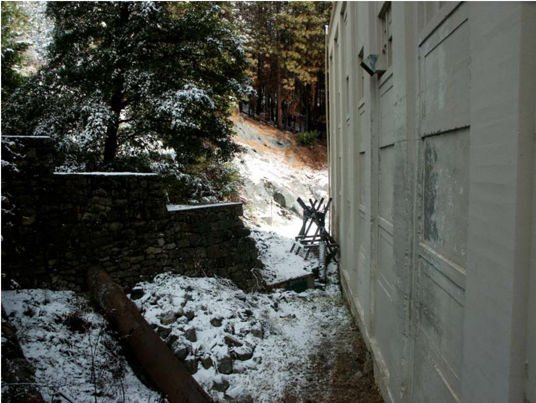
Photo C-3 – Powerhouse No. 1. This photograph taken along the side of Powerhouse No. 1 shows that the hillside area immediately adjacent to the structure is cleared of brush and woody debris. Trees adjacent to the building have been limbed back to provide a defensible space. The building is of concrete construction providing very good fire protection.
