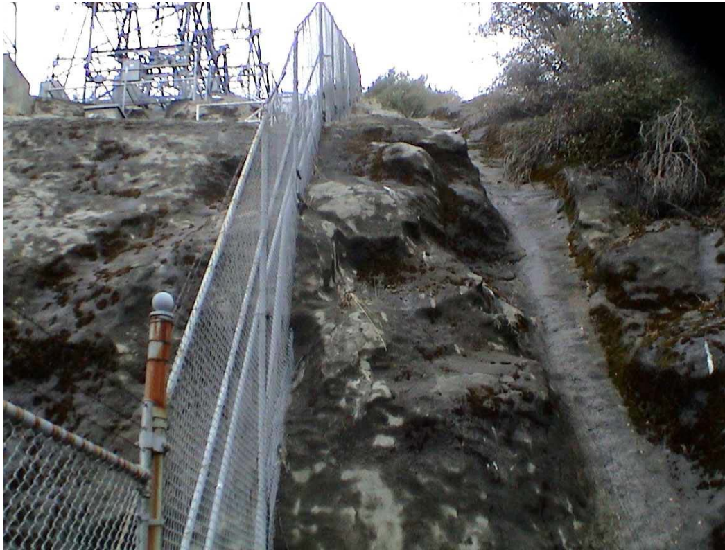
Photo C-12 – Powerhouse 2/2A Switchyard. This photograph shows the clearance of ground fuels and gunite covering within and around the perimeter of switchyard.
