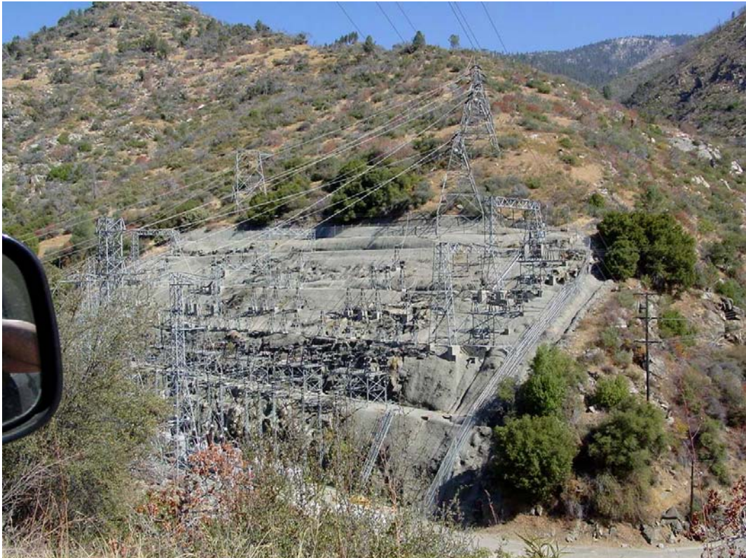
Photo C-11 – Powerhouse 2/2A Switchyard. This photograph shows the cleared area around the perimeter of the switchyard to maintain a defensible space. In addition the ground surface within and around the switchyard is covered with gunite to provide additional fire protection.
