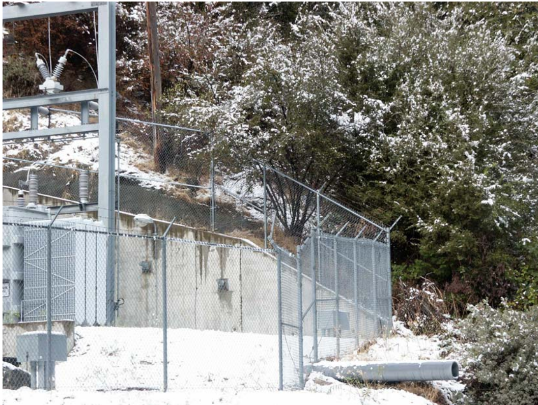
Photo C-6 – Powerhouse No. 1 Switchyard. This photograph shows clearing of ground fuels along the perimeter of the facility. One tree is overhanging the perimeter fence and should be limbed.
